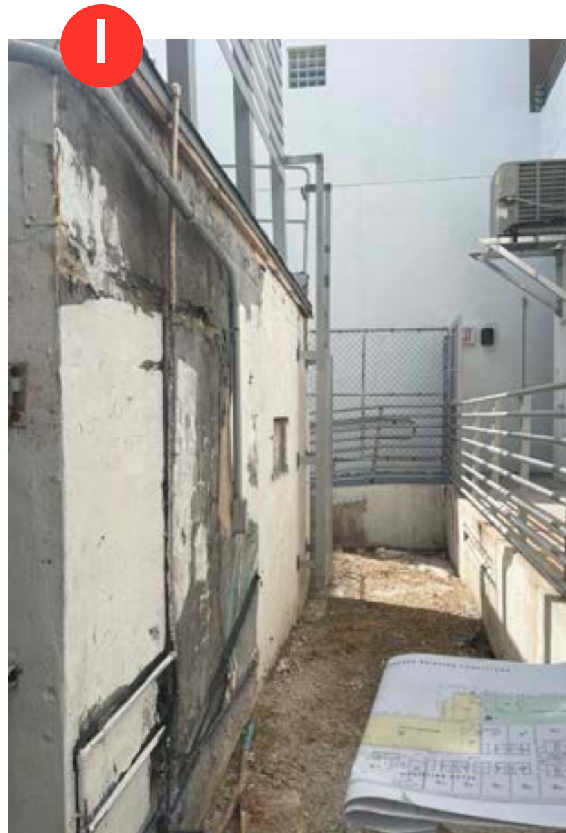
VIEW OF EXISTING MECHANICAL SCREEN ON ROOF NEXT TO Z' OCEAN HOTEL FACING HENROSA'S NORTH PROPERTY LINE
