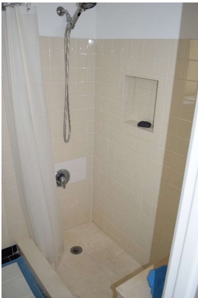
Figure 24. Yellow wall tile at Bath 1, May 2021.
