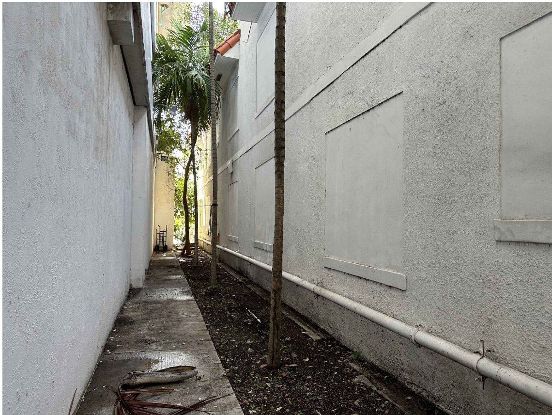
A1 NORTHERN BUILDING FACADE (PUBLIC GARAGE/COMMERCIAL BLDG. ADJACENT TO THE LEFT) PHOTO TAKEN: 06-20-2023
