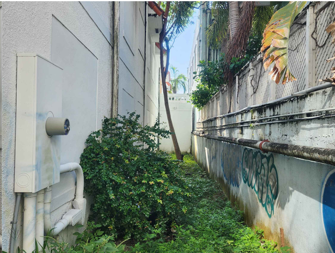
A4 SOUTHERN BUILDING FACADE (COMMERCIAL - MIXED USED BLDG. ADJACENT TO THE RIGHT) PHOTO TAKEN: 06-20-2023
