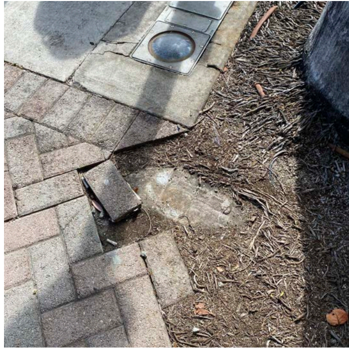
LOOSE CONCRETE PAVERS
