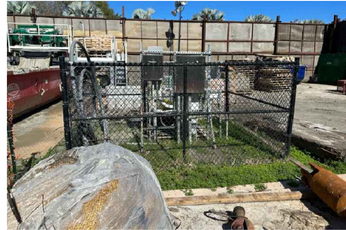
18. ELECTRICAL PANELS IN THE MIDDLE OF FPL STAGING AREA
