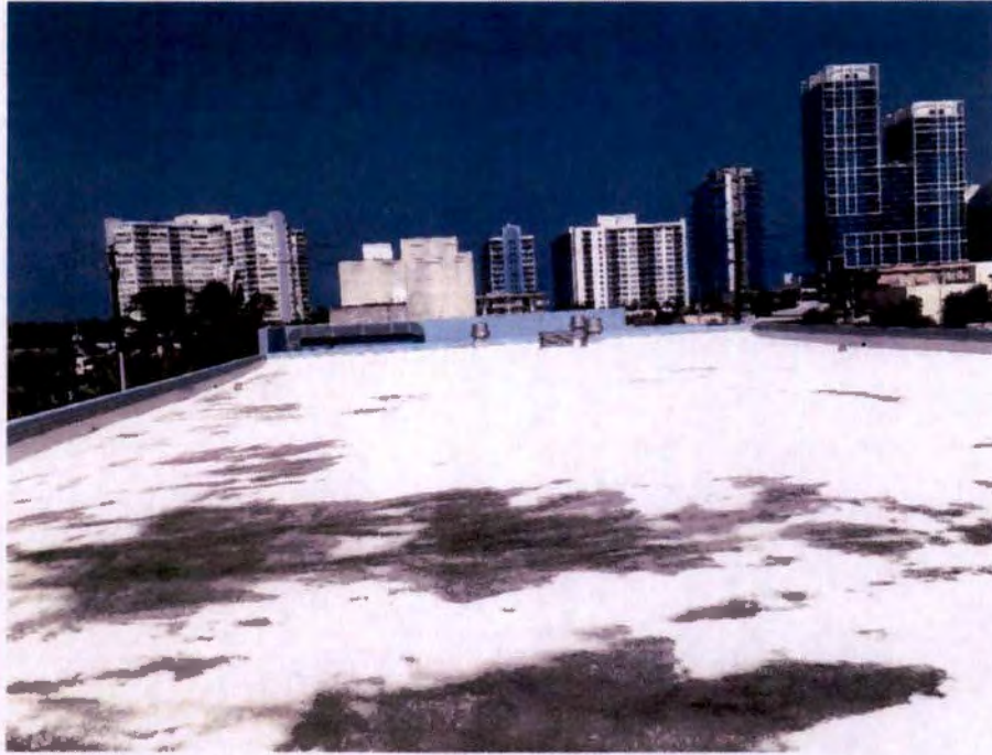
Photograph No. 27 – Deteriorated roofing at Western Upper Roof
