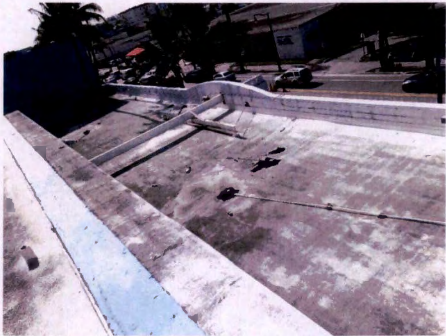
Photograph No. 48 – Low Roof at Second Level in North Portion of Building
