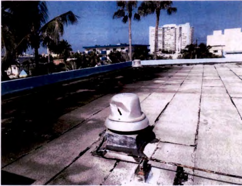
Photograph No. 25 – Deteriorated roofing at Western Upper Roof
