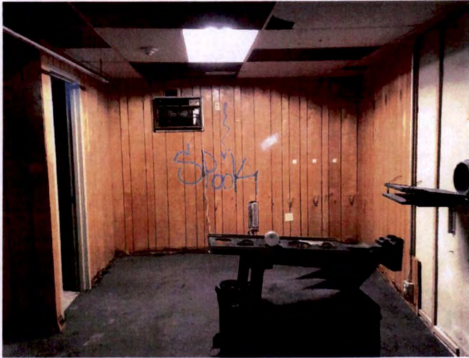
Photograph No. 39 – Deteriorated Interior Wood Paneling in 2 nd floor Room at the South End of Building (Between east and West Theaters).
