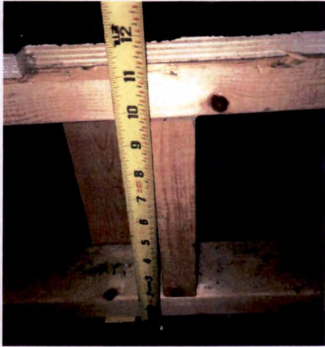
Photograph No. 9 – Built-up Wood Framing over Stage Platform for East Cinema Theater
