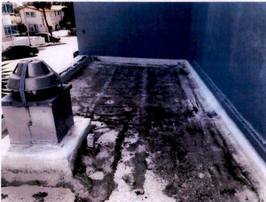
Photograph No. 24 – Deteriorated roofing at Lower Roof at the 2 nd Floor towards South Façade
