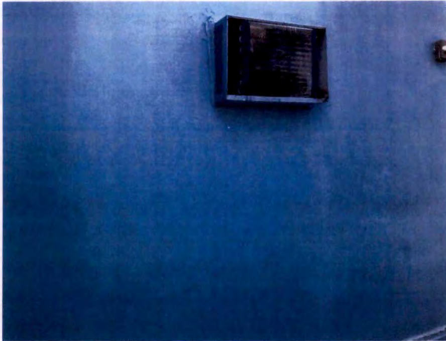
Photograph No. 17 – Uncovered Air Conditioning Unit in 2 nd floor Room at the South End of Building (Between east and West Theaters).
