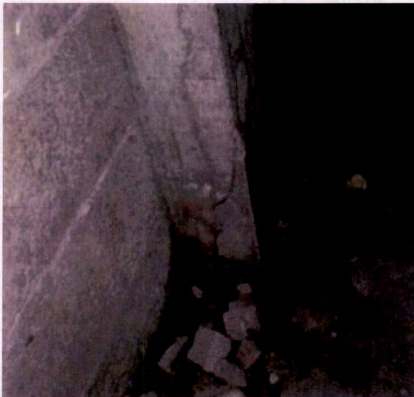
Photograph No. 12 - Spalled Concrete Column at Underground Hall
