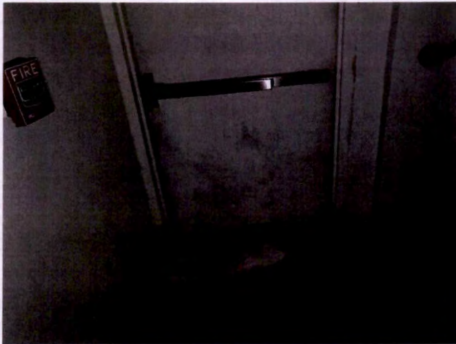
Photograph No. 76 – Corroded Exterior Door at Underground Electrical Room
