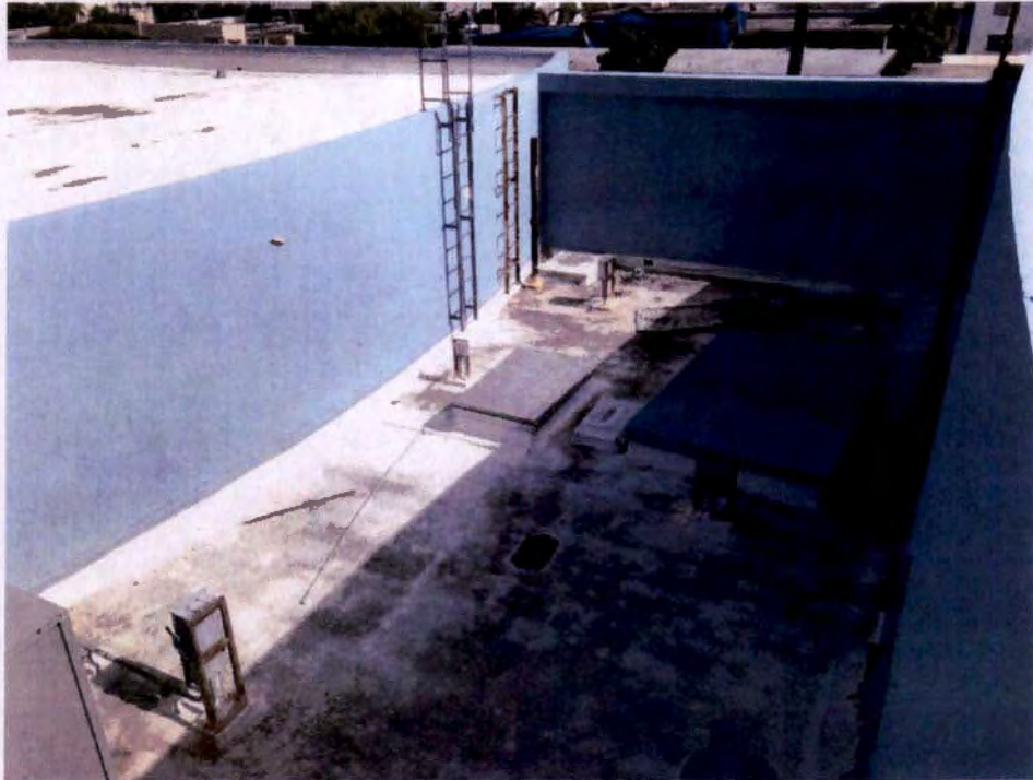
Photograph No. 46 – Lower roof between the East and West Portions of Building
