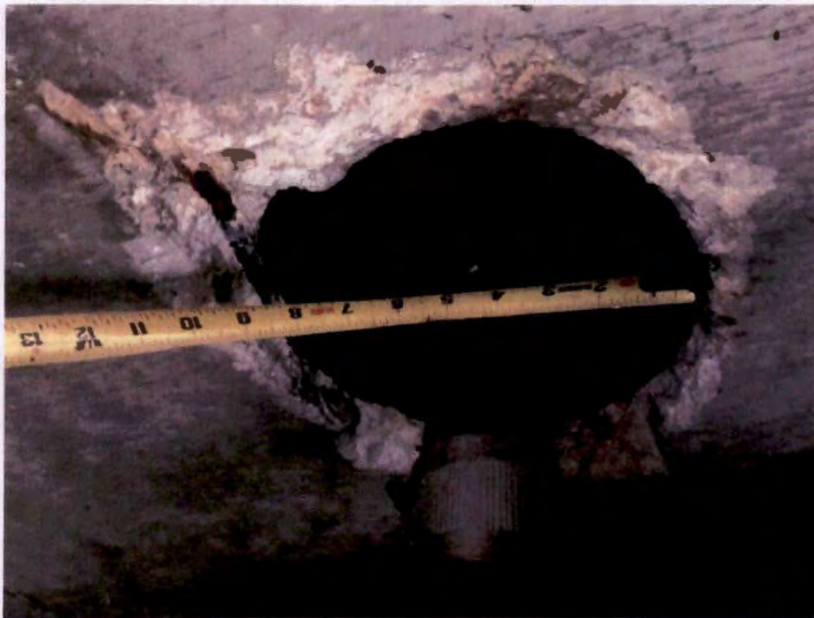
Photograph No. 16 – Opening in Slab above Men's Restroom (near South Façade)
