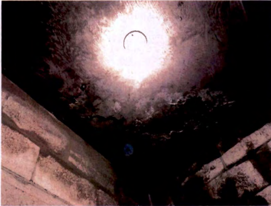
Photograph No. 13 – Spalled Concrete Slab above Electrical Room at Ground Floor
