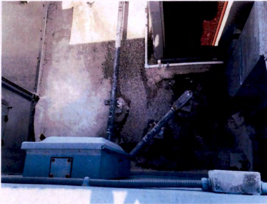
Photograph No. 23 – Deteriorated roofing at Eastern Lower Roof
