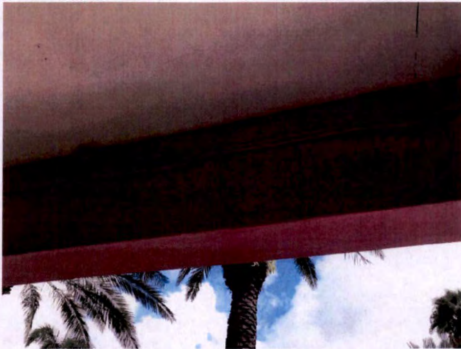
Photograph No. 14 – Spalled Exterior Concrete Beam at North Façade
