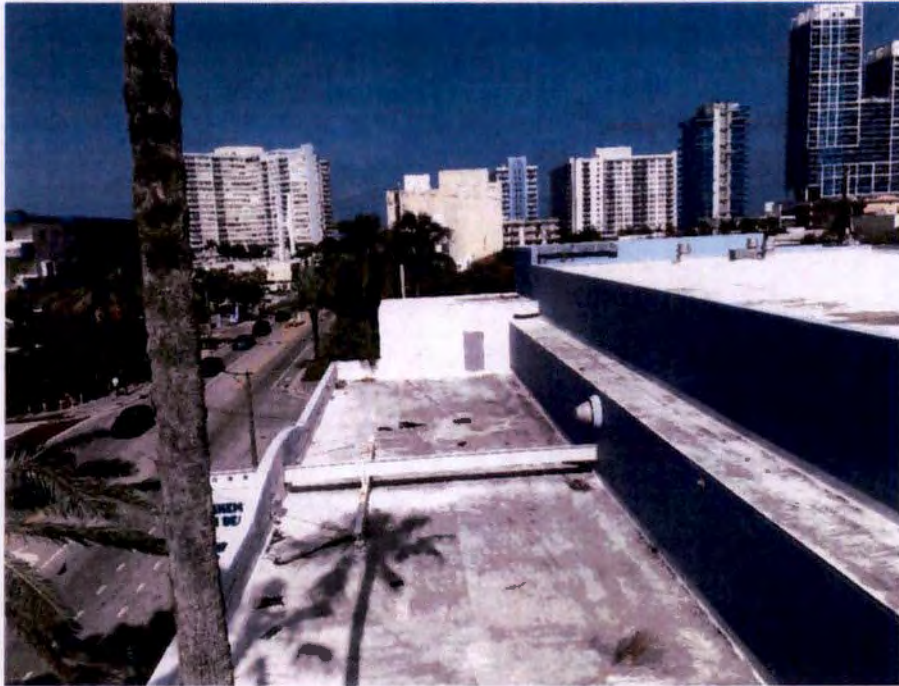
Photograph No. 51 – Low Roof at Northeast Corner of Building and Adjacent Hallway
