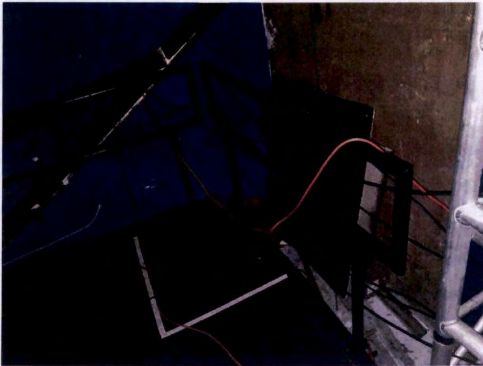
Photograph No. 38 – Loose Metal Guardrail at East Cinema Theater
