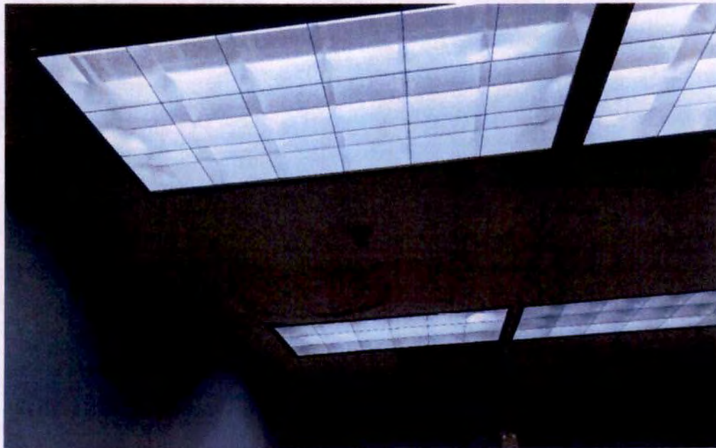
Photograph No. 40 – Stained Ceiling Tiles at Ceiling of First Level
