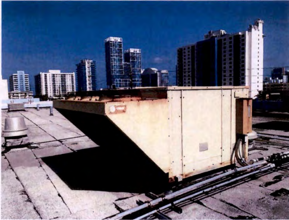
Photograph No. 21 - Rooftop Package Unit at Western Upper Roof
