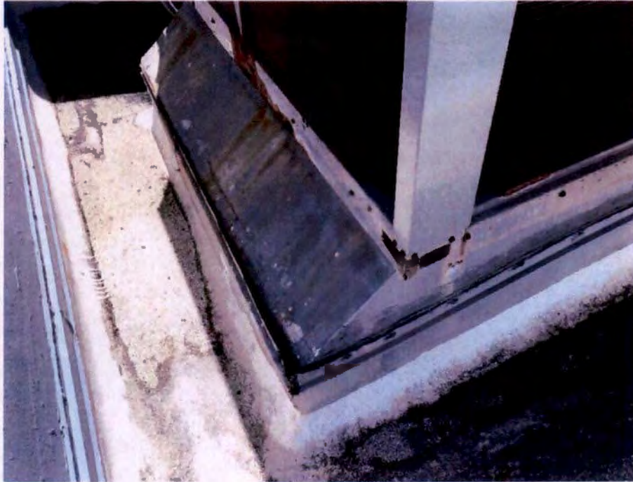
Photograph No. 65 – Package Unit Unconnected to Roof Curb at Low Roof between East and West Portions
