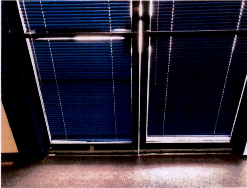
Photograph No. 75 – Considerable Gab between Pair of North Façade Doors
