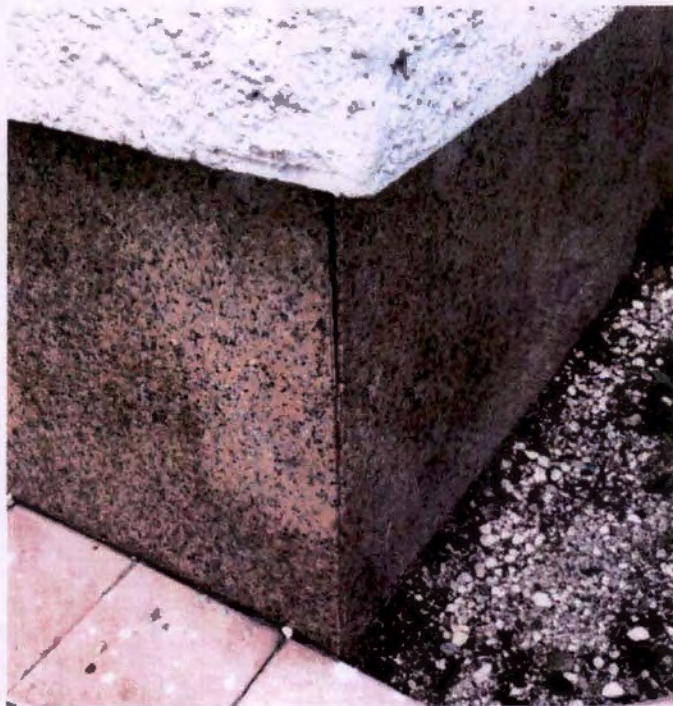
Photograph No. 30 – Gap at Exterior Tile at Northeast Corner
