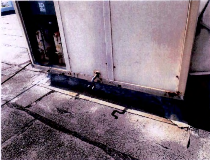
Photograph No. 63 – Package unit Unconnected to Roof Curb at Western Upper Roof
