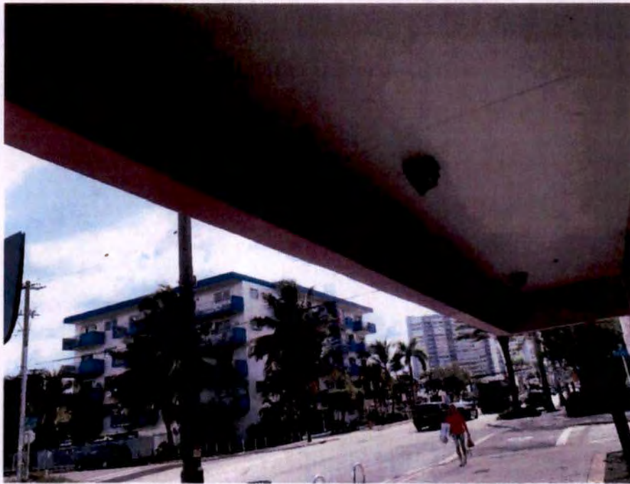
Photograph No. 15 – Spalled Exterior Concrete Beam at North Façade
