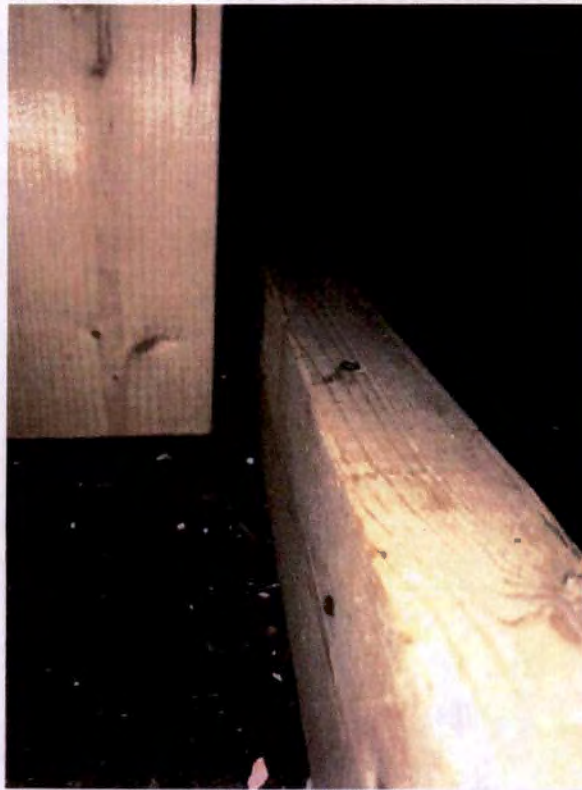
Photograph No. 36 – Gap between vertical member and bottom plate
