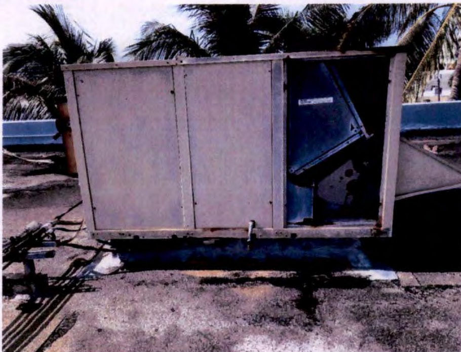
Photograph No. 64 – Package unit Unconnected to Roof Curb at Western Upper Roof
