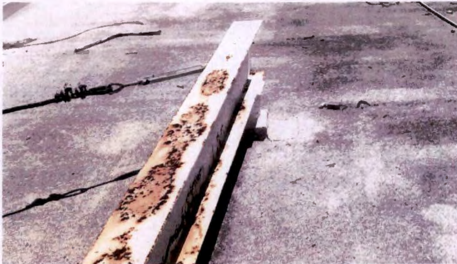
Photograph No. 20– Corroded Structural Steel Supporting Theater Sign
