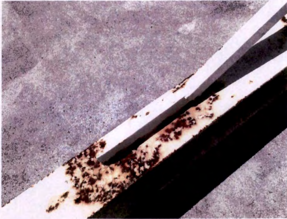
Photograph No. 19 – Corroded Structural Steel Supporting Theater Sign
