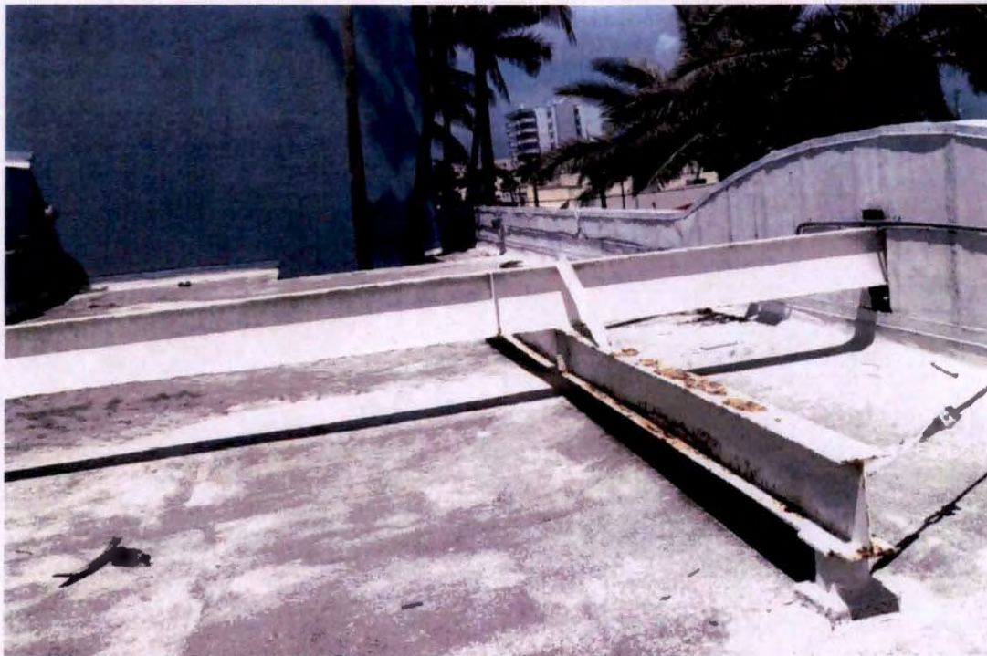
Photograph No. 18 – Corroded Structural Steel Supporting Theater Sign
