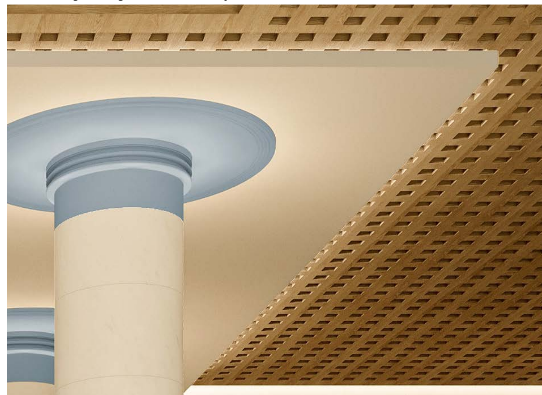
Cove lighting at drop ceiling
