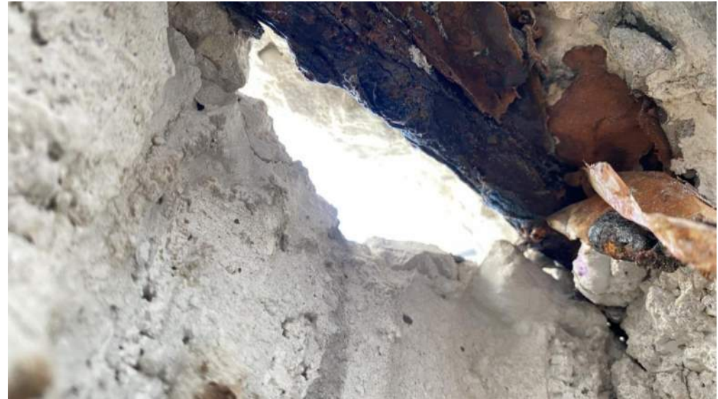
Unbonded concrete and corroded reinforcement
