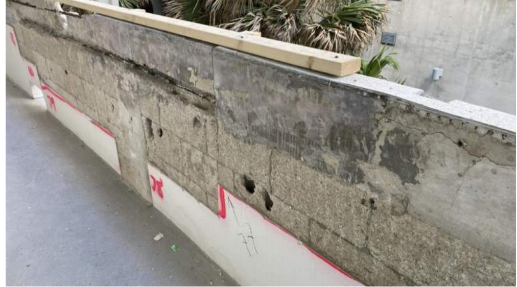
Distressed concrete and exposed / corroded reinforcement
