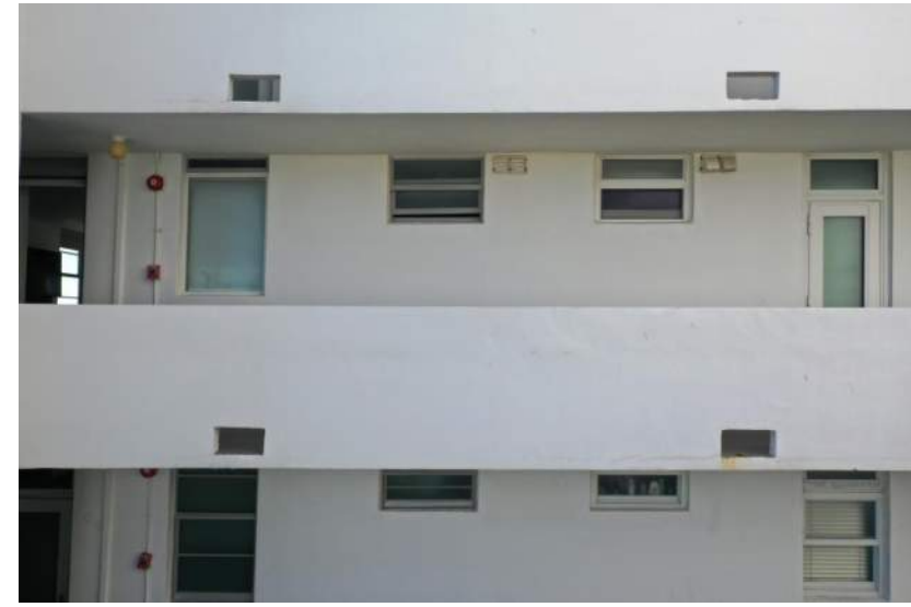
Existing Catwalk Guardrails
