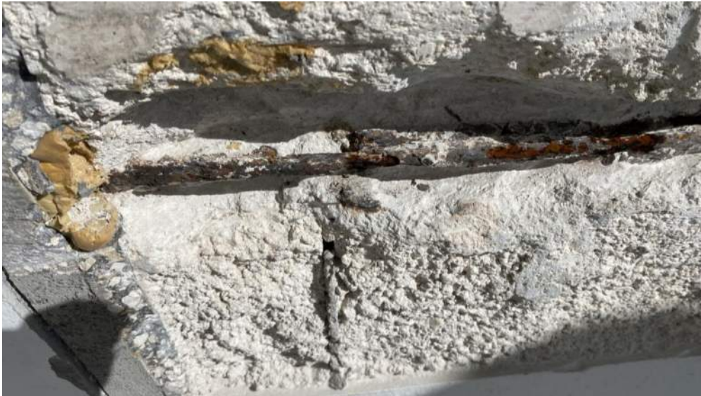
Unbonded concrete and corroded reinforcement
