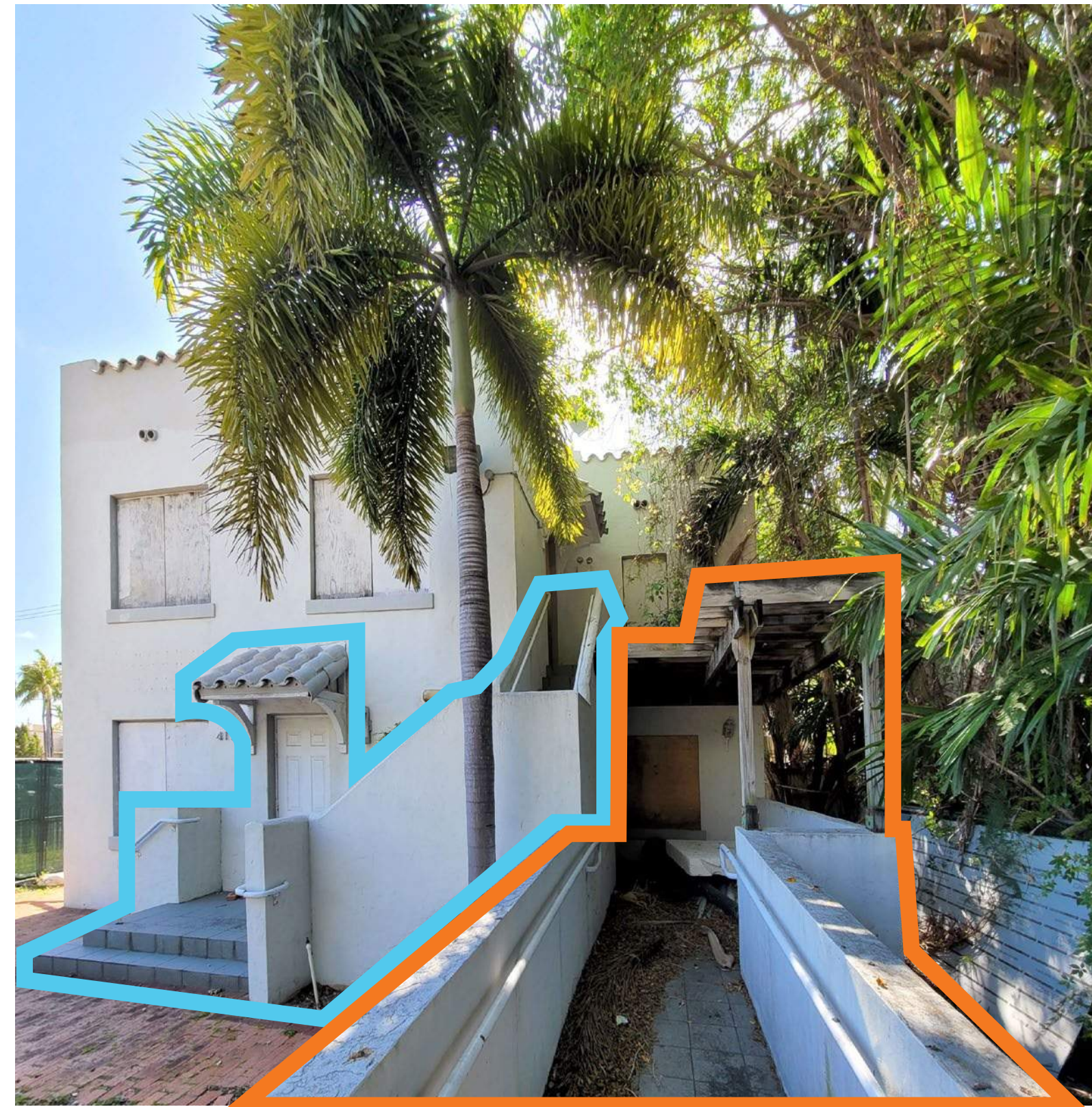
FRONT ENTRY STAIR - TO BE REPLACED
