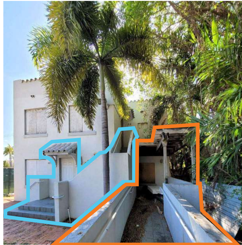
FRONT ENTRY STAIR - TO BE REPLACED
