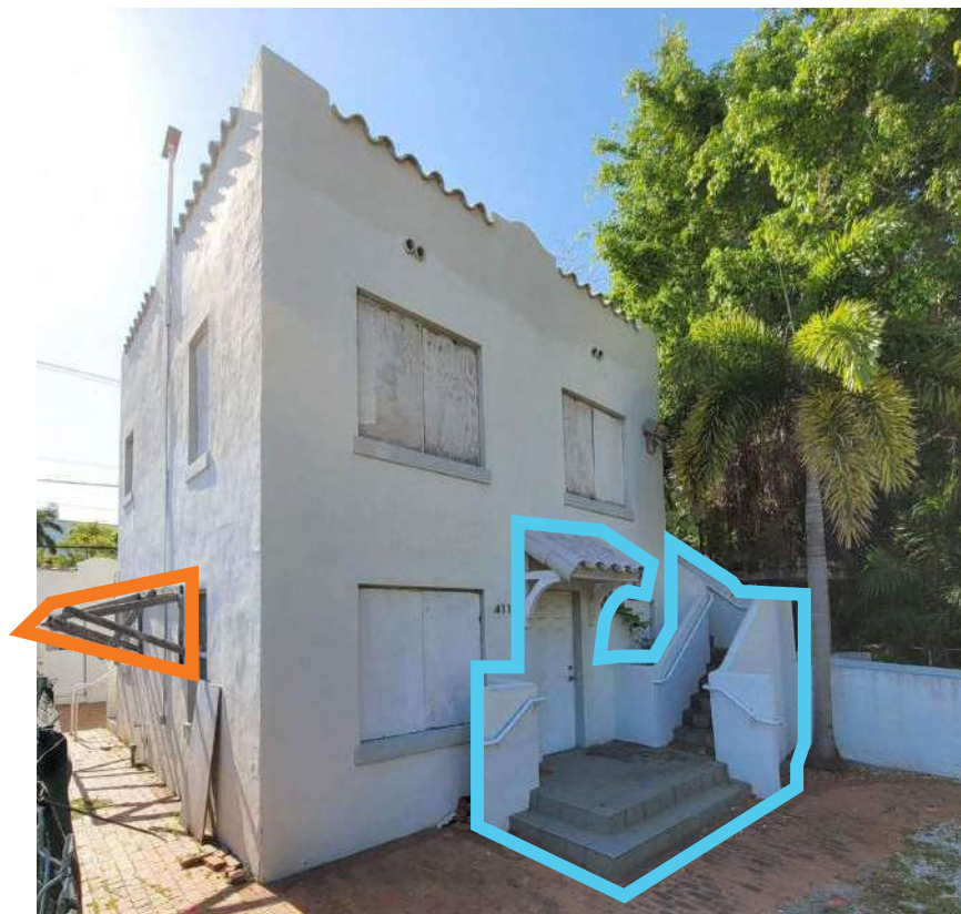
WOOD TRELLIS - TO BE REMOVED FRONT ENTRY & STAIR - TO BE REPLACED
