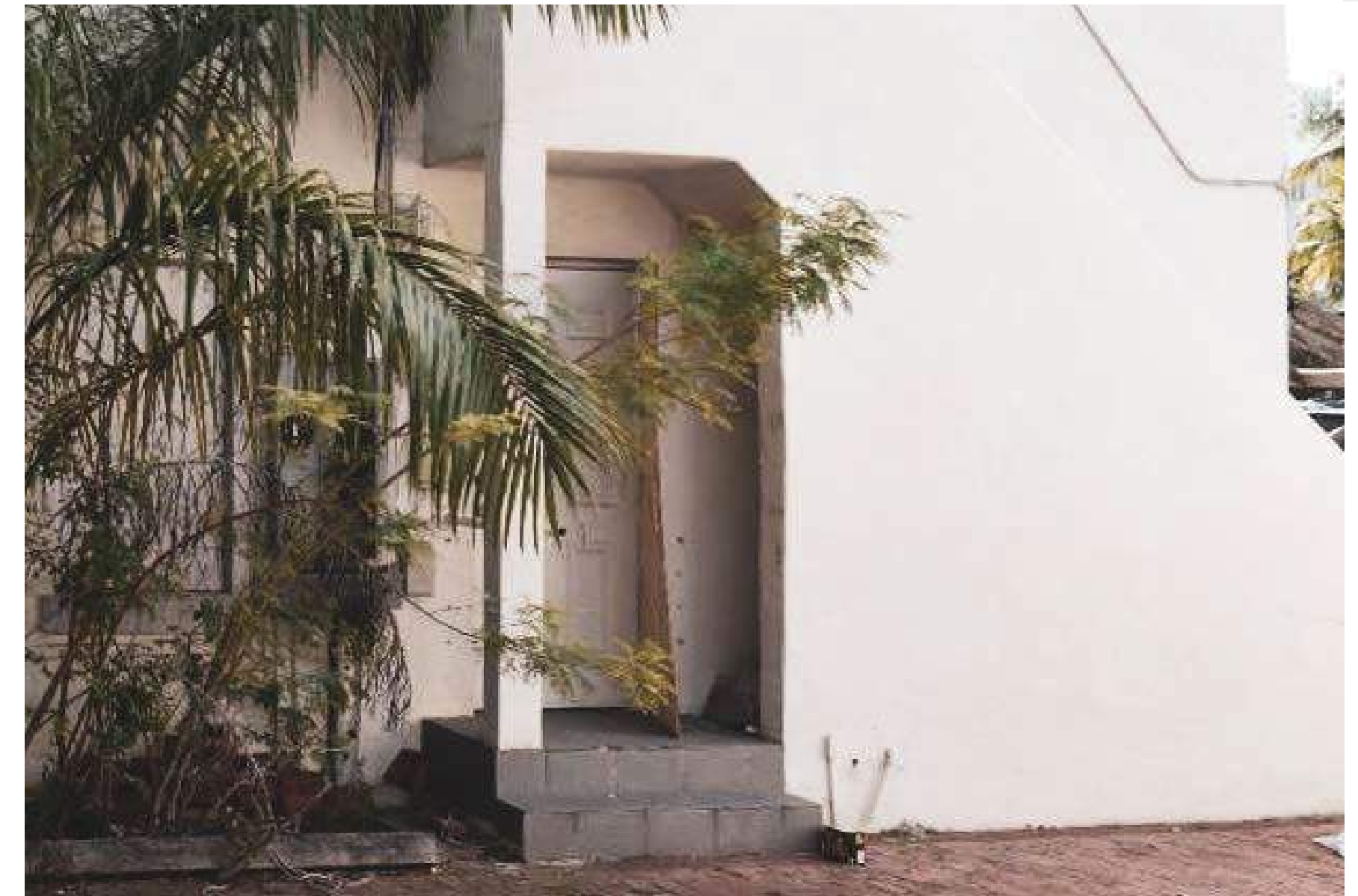
1st Level Detail NON-ORIGINAL DOOR OPENING (TO BE REMOVED)
