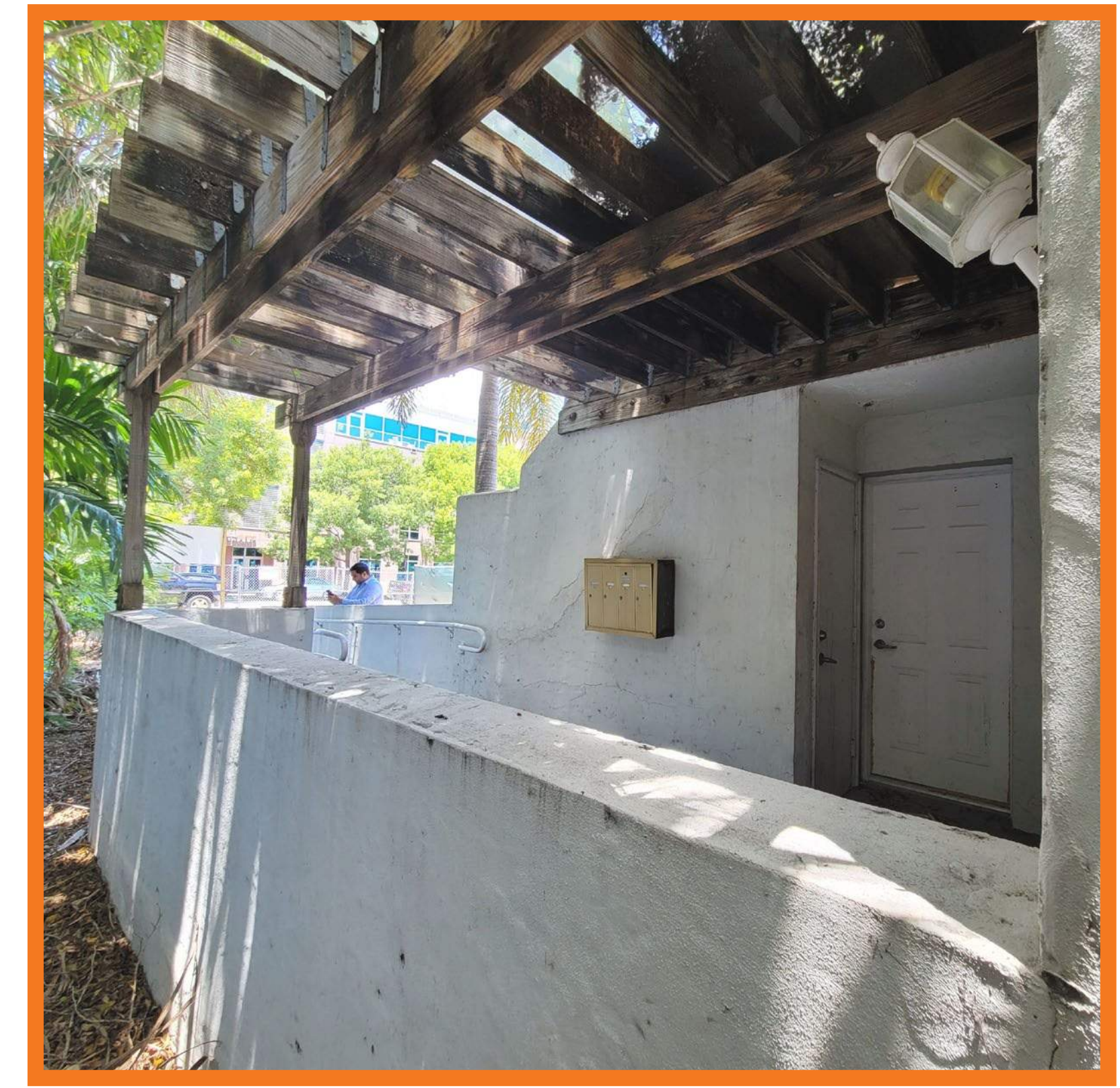
ACCESS RAMP AND WOOD TRELLIS - NOT ORIGINAL (2001) TO BE REMOVED
