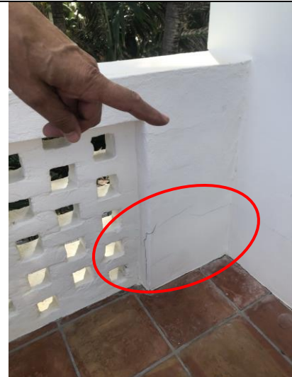
Concrete crack on the balcony
