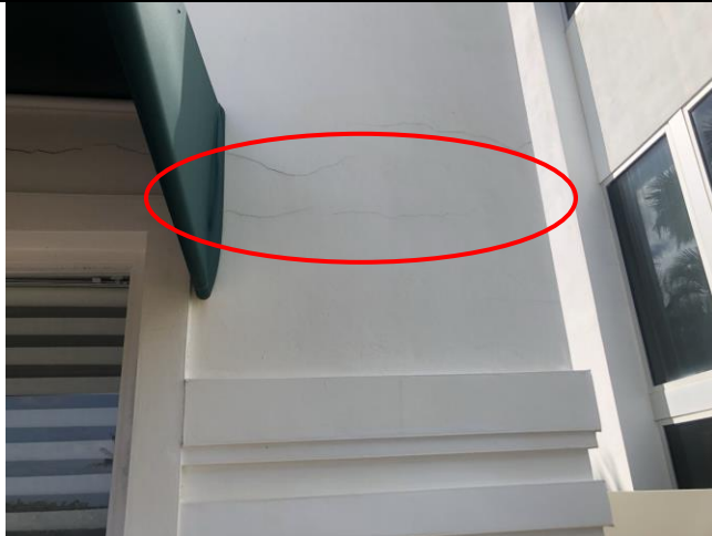
Linear crack on the corner
