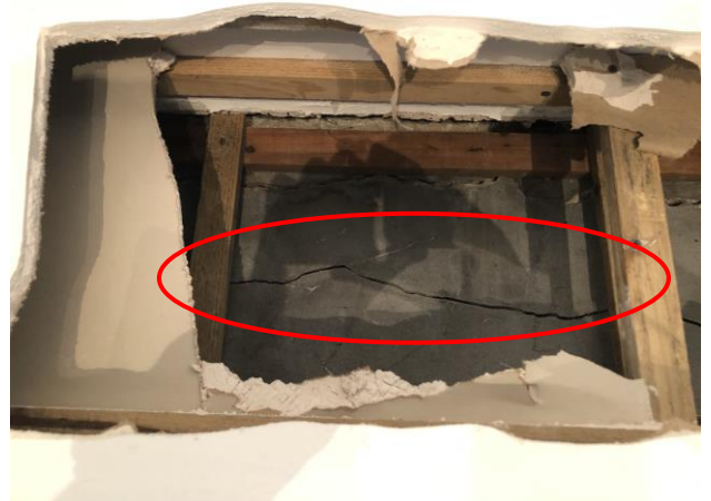
Critical Linear Crack on the lintel beam
