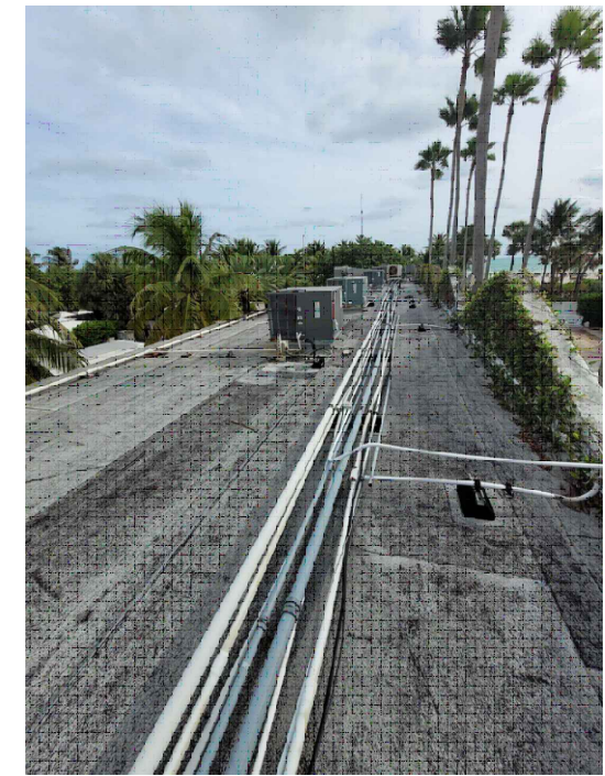
PHOTO OF EXISTING ROOFTOP MECHANICAL EQUIPMENT
