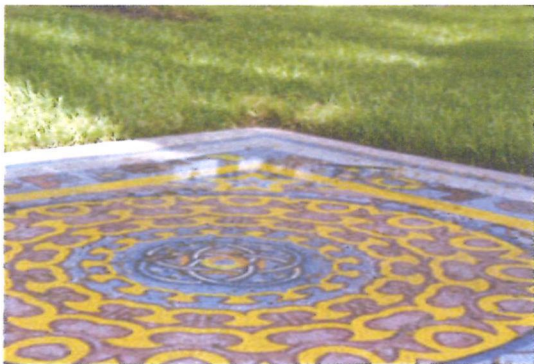
Standing water on southeast side of the mosaic.
