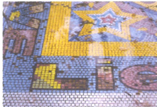
Detail of pooling water with visible algae on the grout and in areas where tiles have been displaced. .
