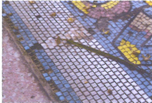
Detail of tile loss, standing water, dirt, and debris sitting on the mosaic
