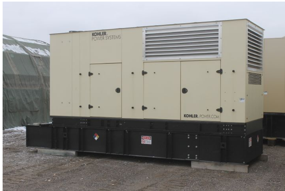
SIMILAR GENERATOR - FRONT ANGLE WITH FUEL TANK
