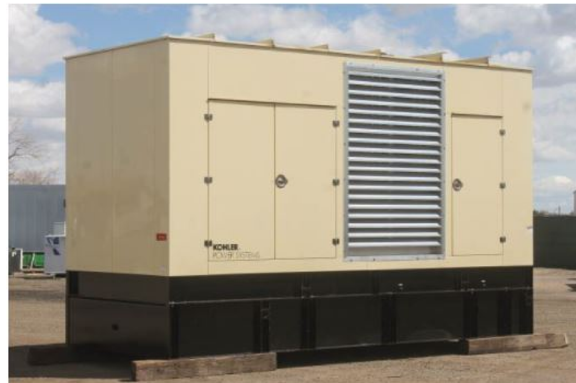
SIMILAR GENERATOR - REAR ANGLE WITH FUEL TANK
