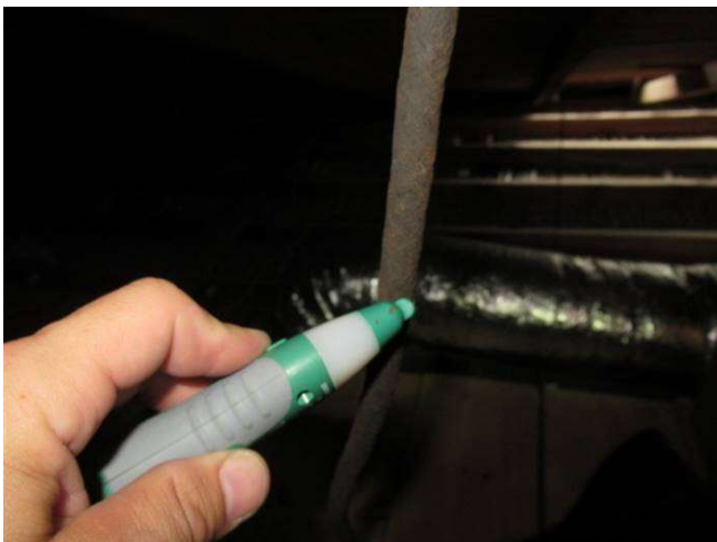
ABANDONED CLOTH WIRING
