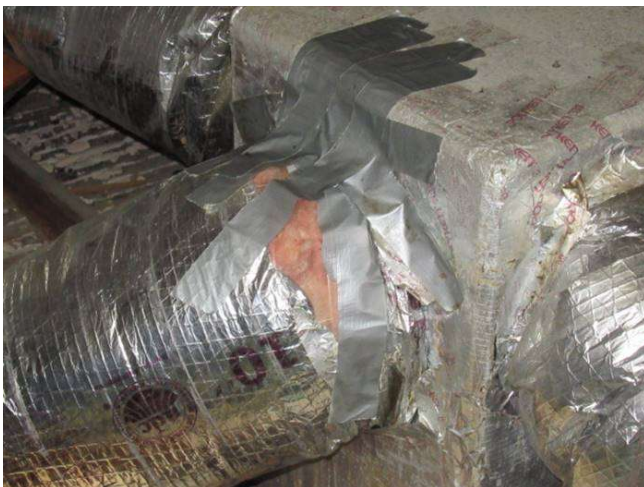
TORN DUCT WORK
