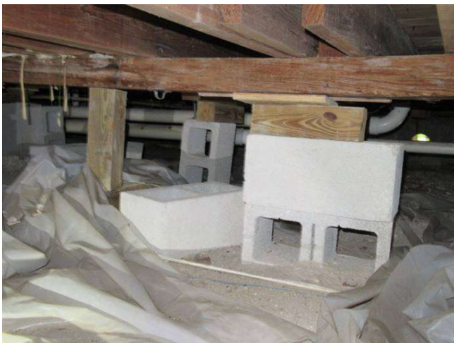
IMPROPER SUBFLOOR SUPPORTS
