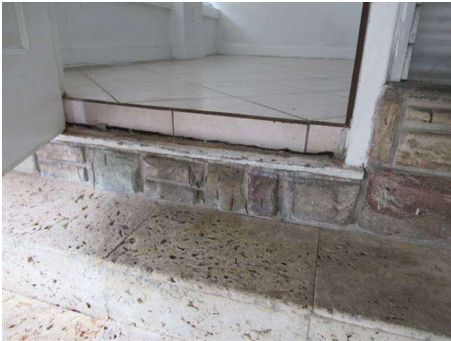
IMPROPER STEP HEIGHT
