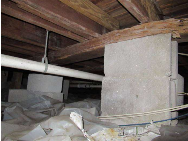
CRACKED SUBFLOOR BEAMS
