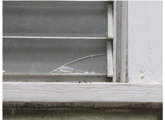
CRACKED JALOUSIE PANE
