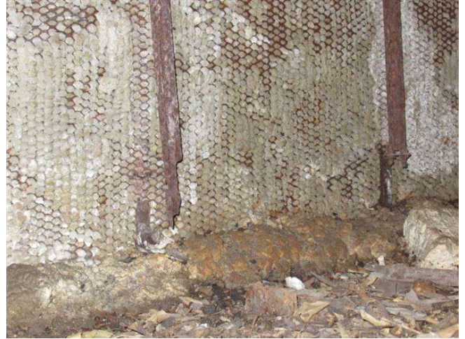
CORRODED WALL FRAMING
