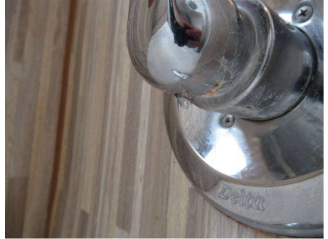
LEAKING SHOWER HANDLE
