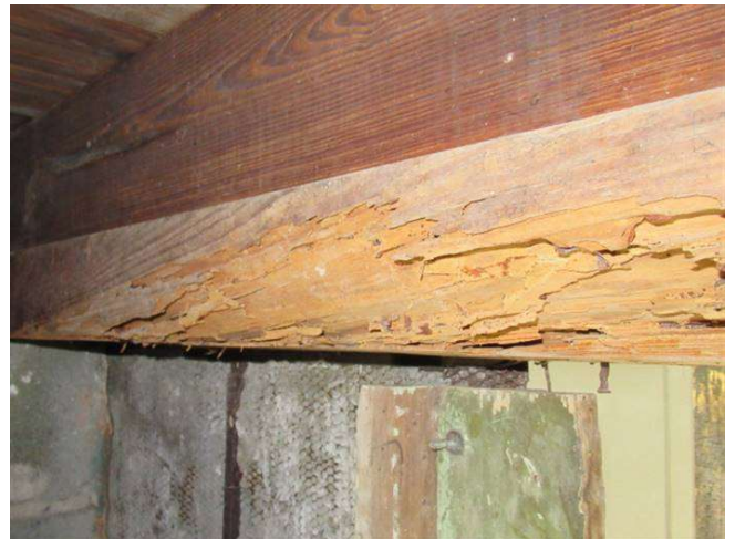
SUBTERRANEAN TERMITE DAMAGE
