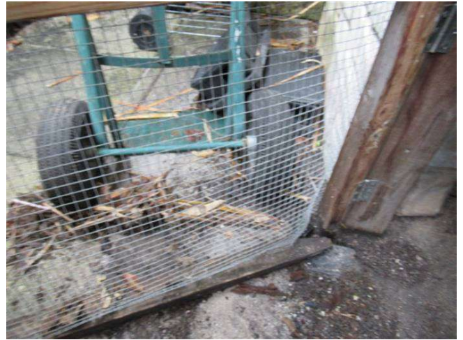
DAMAGED CRAWLSPACE DOOR
