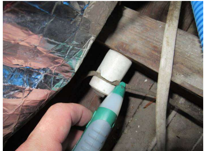
ABANDONED CLOTH WIRING
