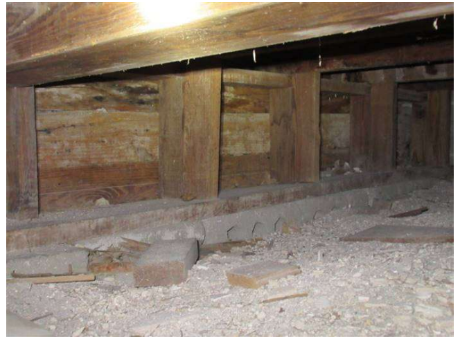
IMPROPER SUBFLOOR SUPPORTS
