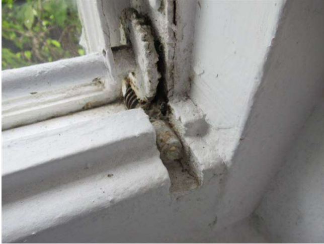
MISSING CRANK HANDLES
