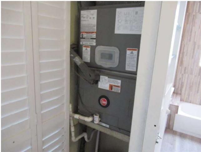
AIR HANDLER UNIT
