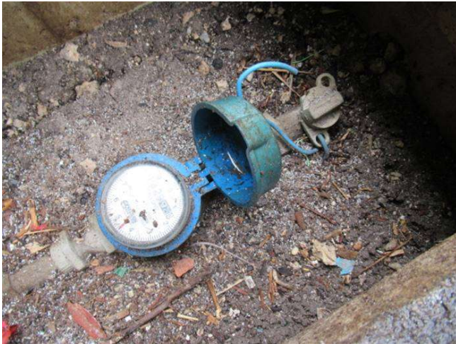
MAIN SHUT OFF VALVE
