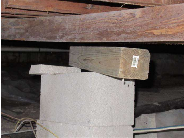
IMPROPER SUBFLOOR SUPPORTS
