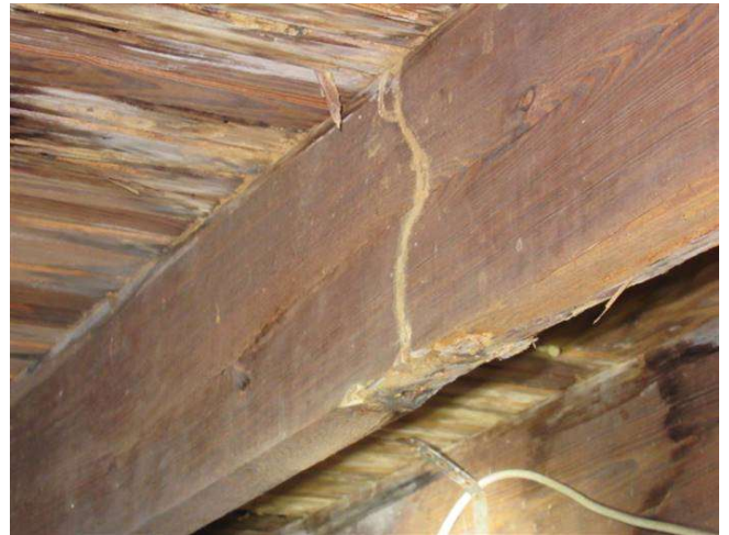
SUBTERRANEAN TERMITE DAMAGE
