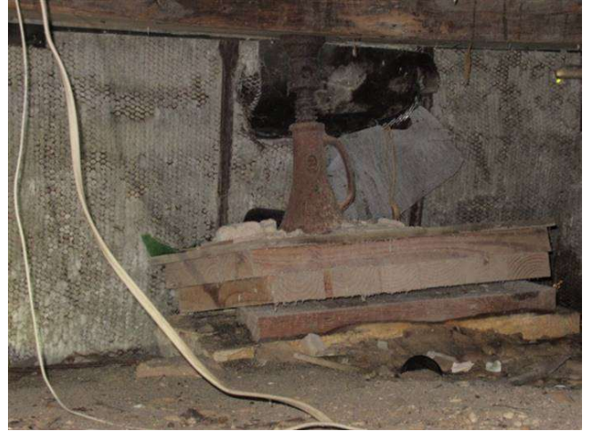
IMPROPER SUBFLOOR SUPPORTS
