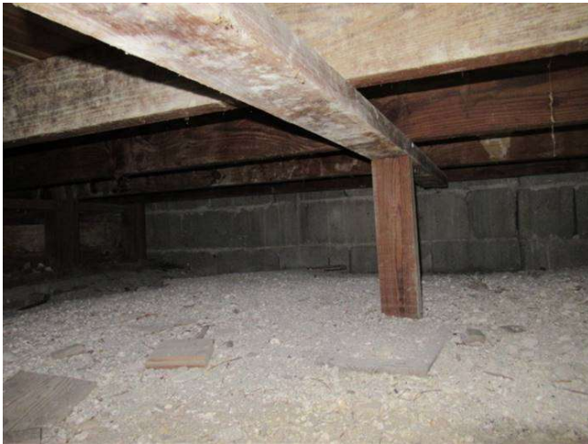
IMPROPER SUBFLOOR SUPPORTS
