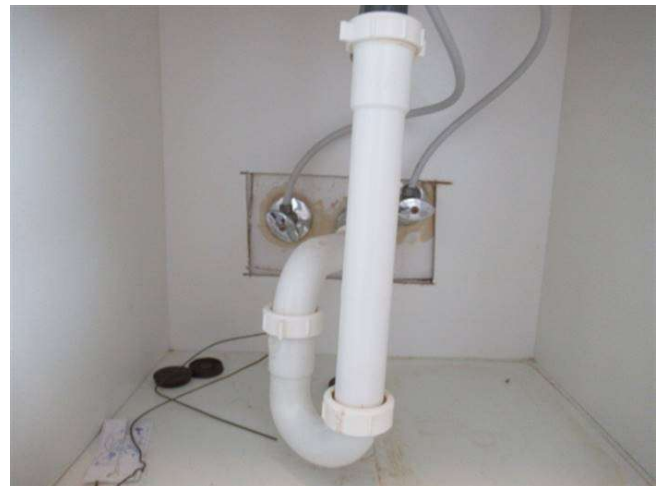
UNDER SINK PIPING
