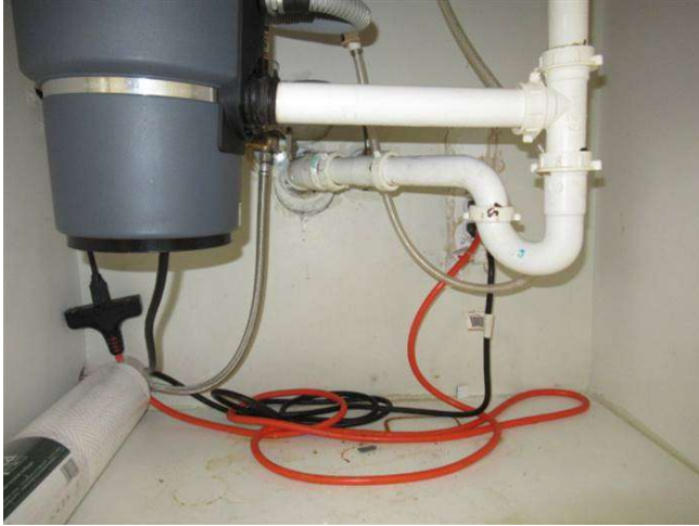
UNDER SINK PIPING
