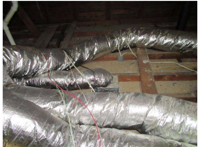
DUCTWORK IS RESTING ON CEILING JOISTS
