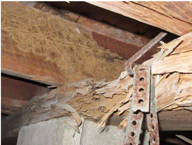
SUBTERRANEAN TERMITE DAMAGE
