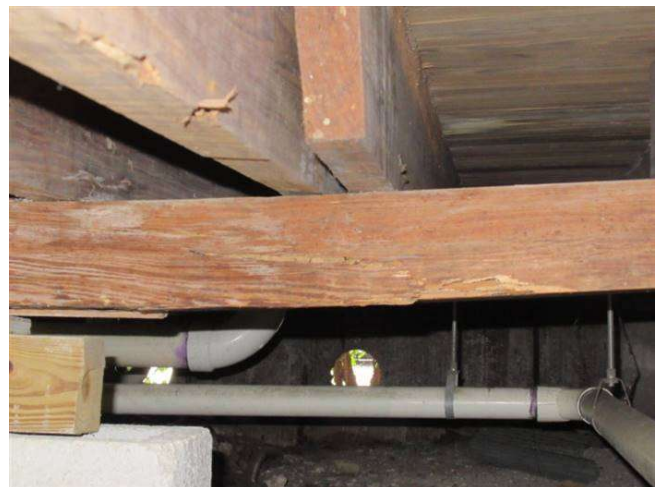
CRACKED SUBFLOOR BEAMS
