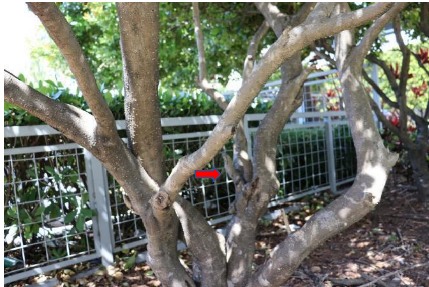
Note shaping, stub cuts (red arrow) and poor structure.
