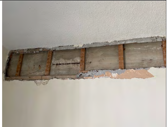
Photo 28 - North elevation concrete spalling and corroded rebar
