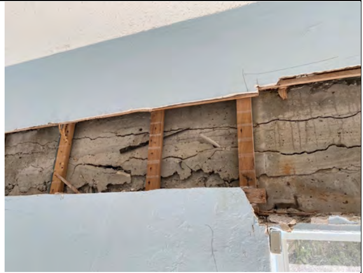
Photo 26 - South elevation concrete spalling and corroded rebar
