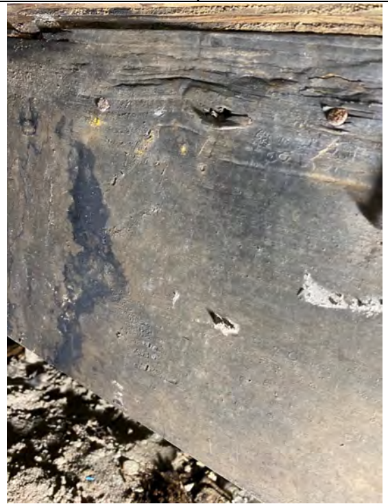
Photo 16 - Crawl space under house showing damaged floor joists
