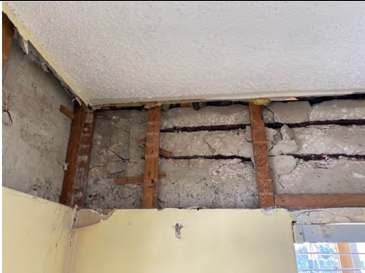
Photo 27 - North elevation concrete spalling and corroded rebar
