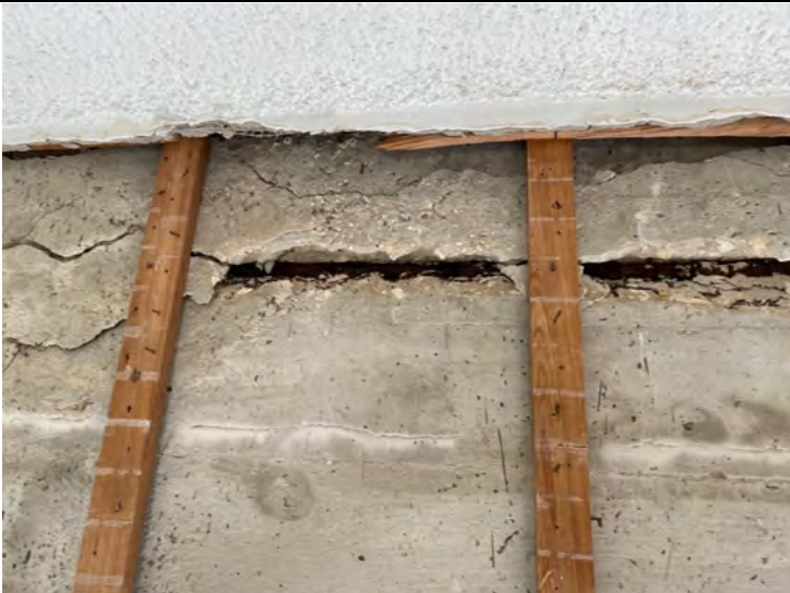
Photo 25 - South elevation concrete spalling and corroded rebar
