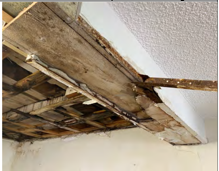
Photo 32 - Covered patio roof damage
