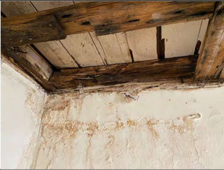
Photo 33 - Covered patio roof damage
