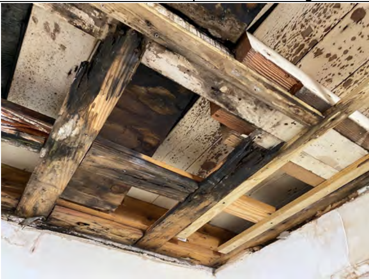
Photo 31 - Covered patio roof damage
