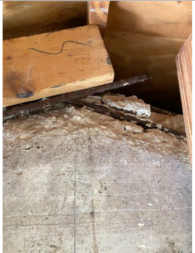
Photo 24 - West elevation concrete spalling and corroded rebar
