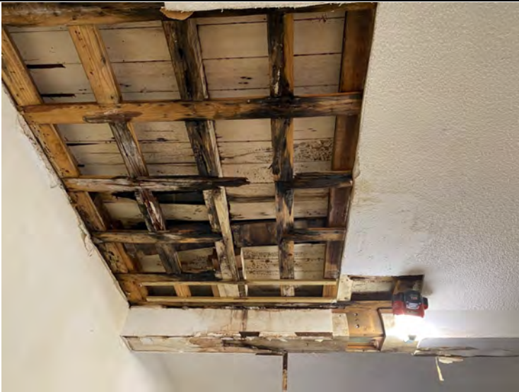
Photo 29 – Covered patio roof damage
