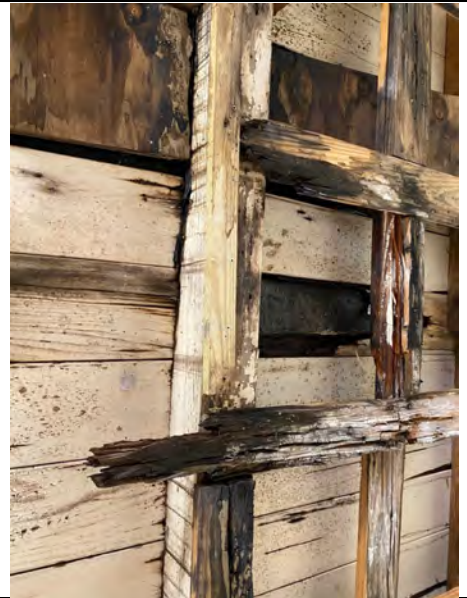
Photo 30 - Covered patio roof damage
