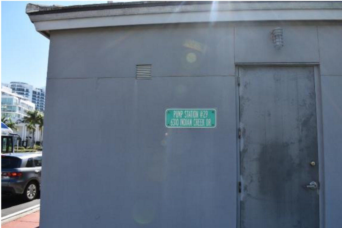
Photo 8 View of identification sign on Pump Station #29
