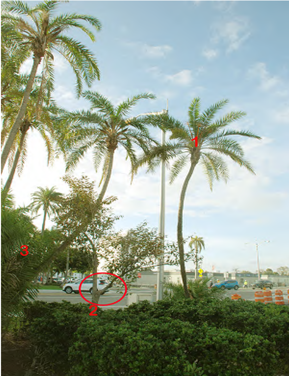
Photo 1 above is palm 1 and tree 2 viewed from the east. Palm 1 has only a single trunk. Tree 2 as indicated by the circle has a very weak trunk/main branch connection.
