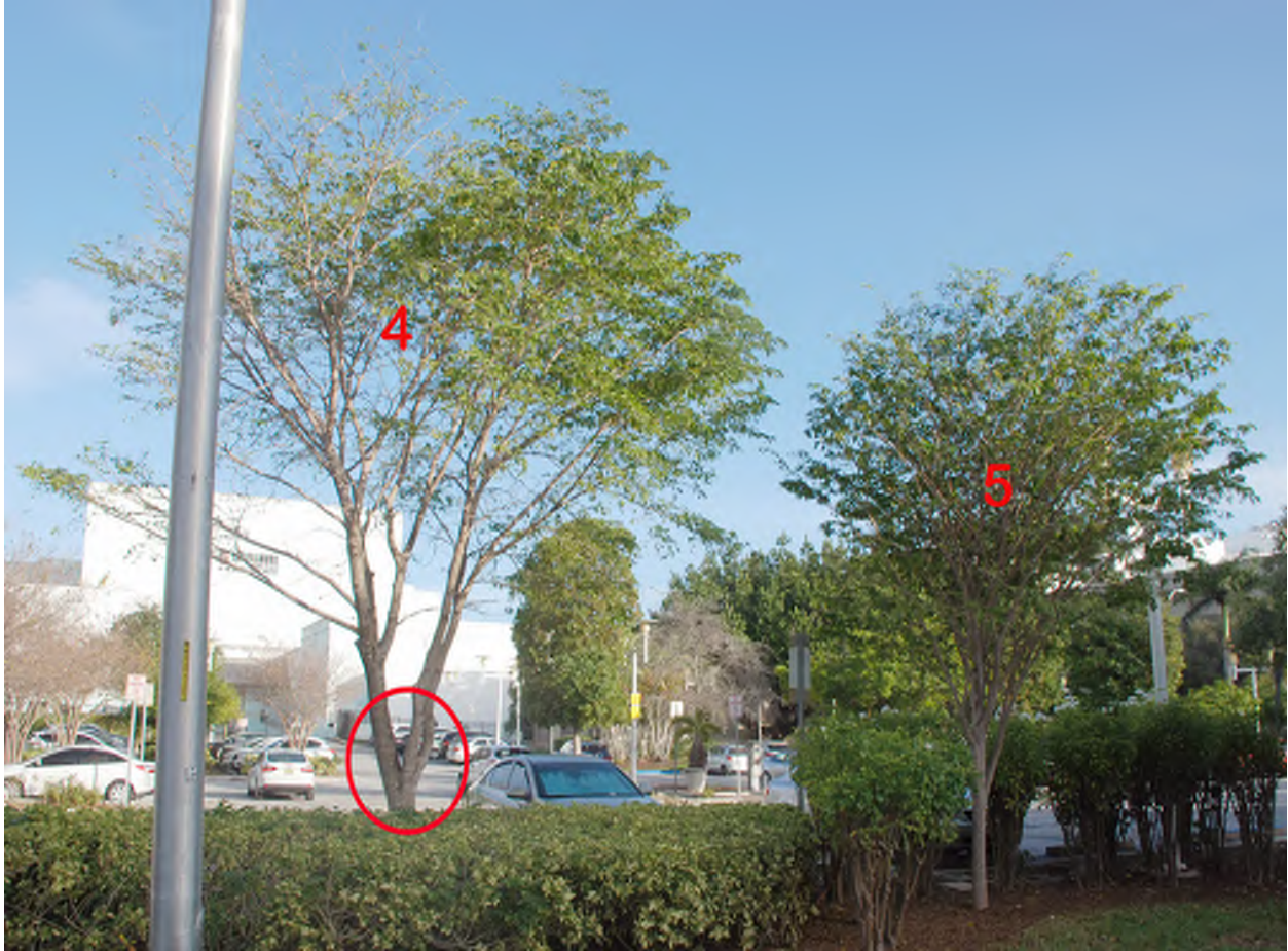
Photo 4 above is tree 4 with the circle indicating a very weak trunk/main branch connection, and tree 5 viewed from the west.
