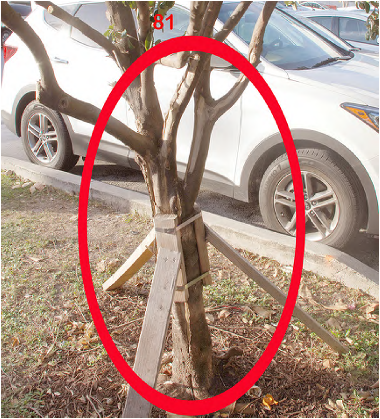
Photo 49 above is a closer view of the damaged trunk of tree 81. This tree should be removed.
