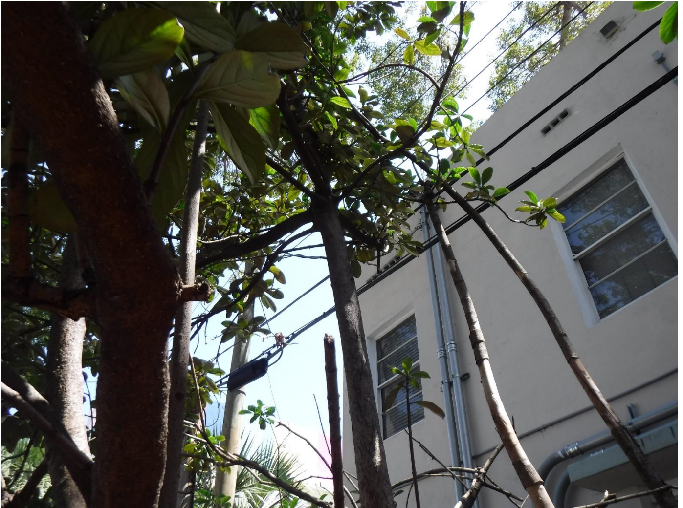
Tree # 41 growing into overhead wires
