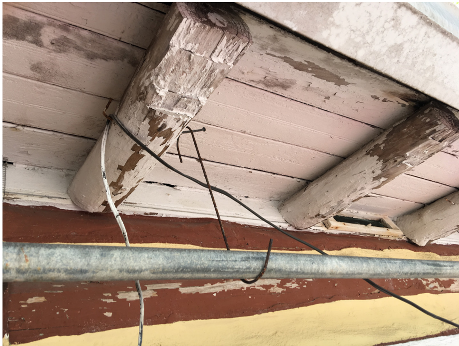
Detail Rotted Wood
