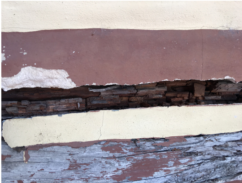
Detail Rotted Wood
