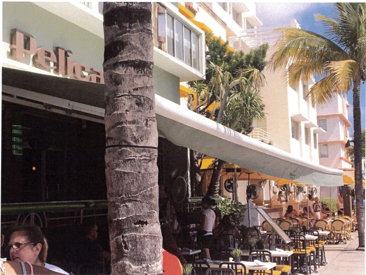
Unpermitted retractable awning, August 2017.
