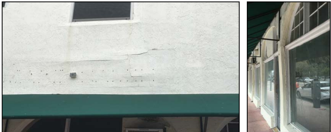
Cracking and Bulging at Exterior Walls
