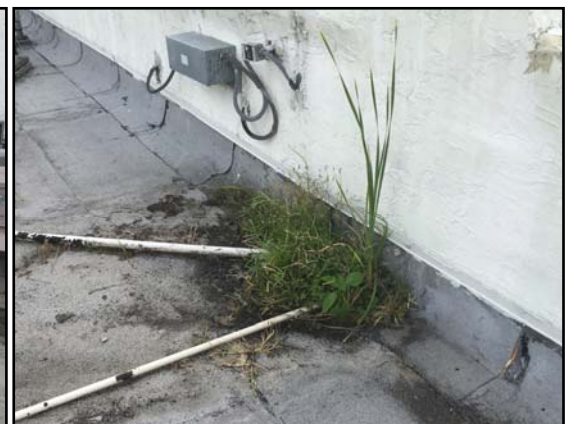
Plant near drainage spot at roof
