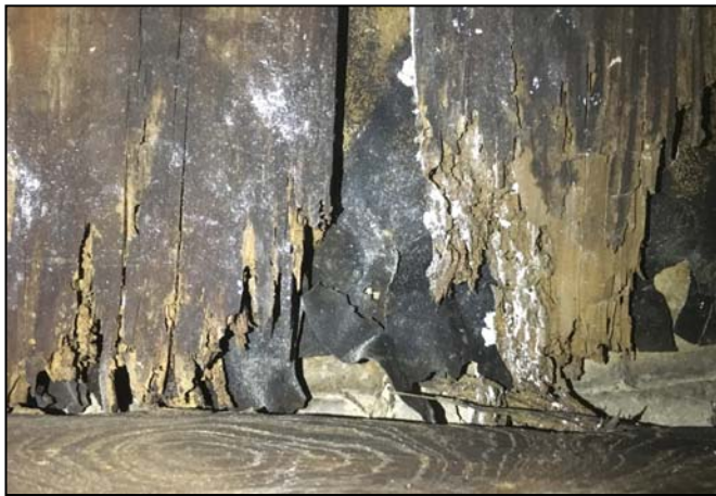
Severe Rotting in Exterior Wood Framed Walls
