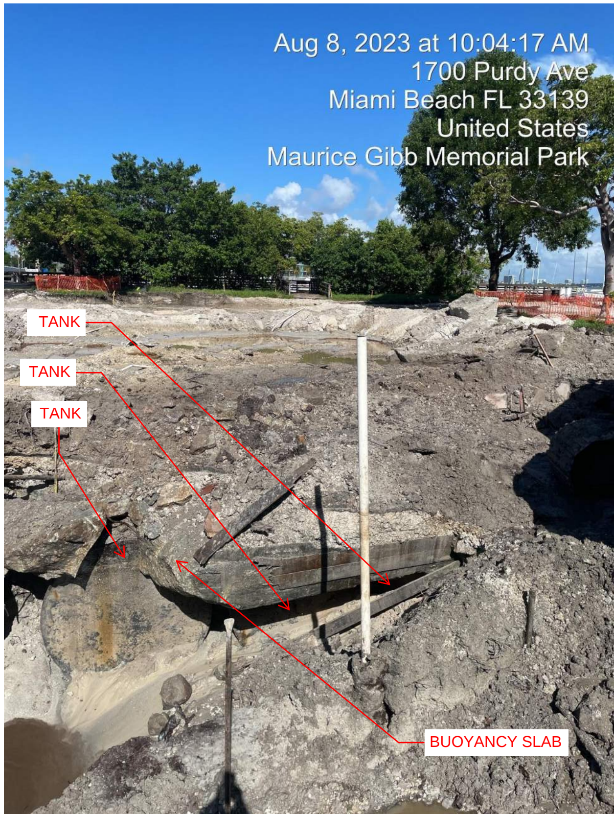
Area D: Underground fuel tank exposed.
