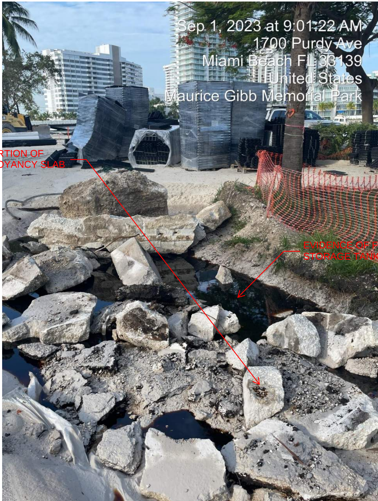
Area E: Concrete slab and footings removed. Fuel encountered signaled possibility of an underground fuel tank.
