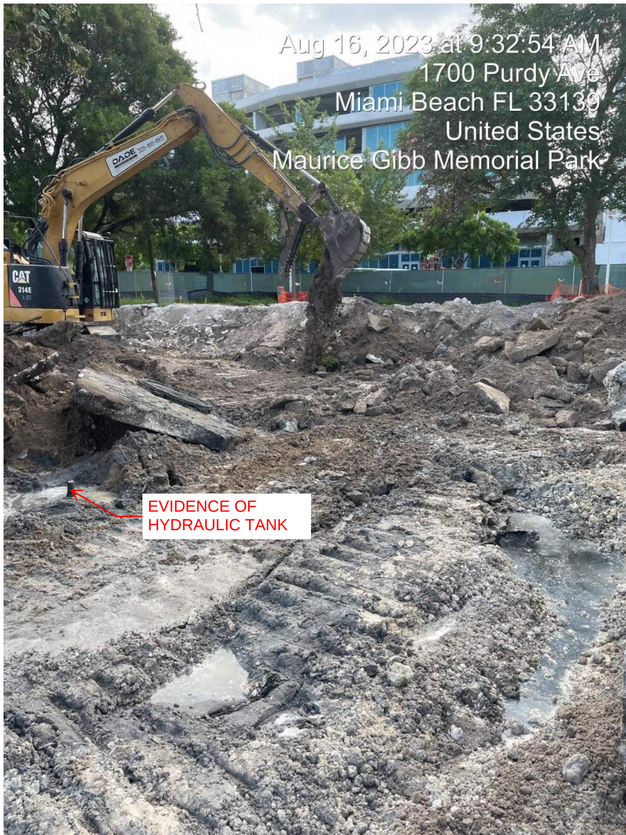
Area F: Hydraulic fuel discovered, adjacent to estimated 20' diameter tank.
