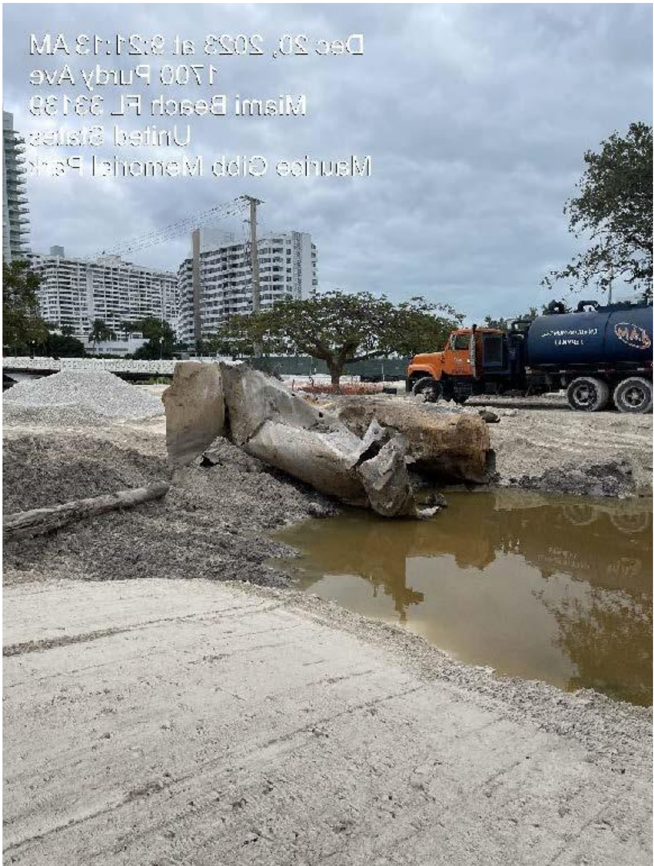
Area D: Unforeseen, underground fuel storage tank removed for the execution of work. Fuel encountered within the ground water was removed.
