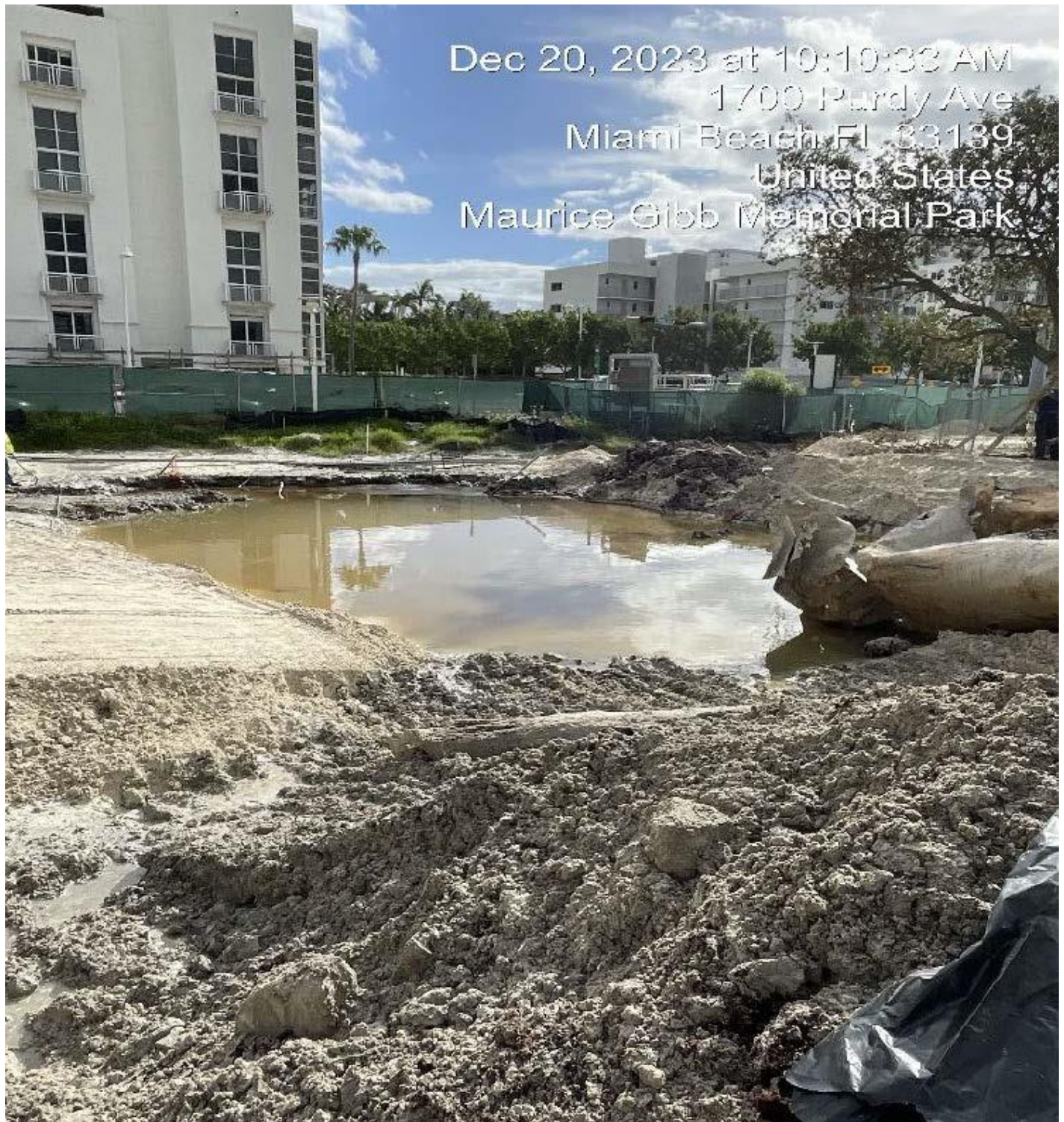
Area D: Unforeseen fuel tanks were encountered and removed.
