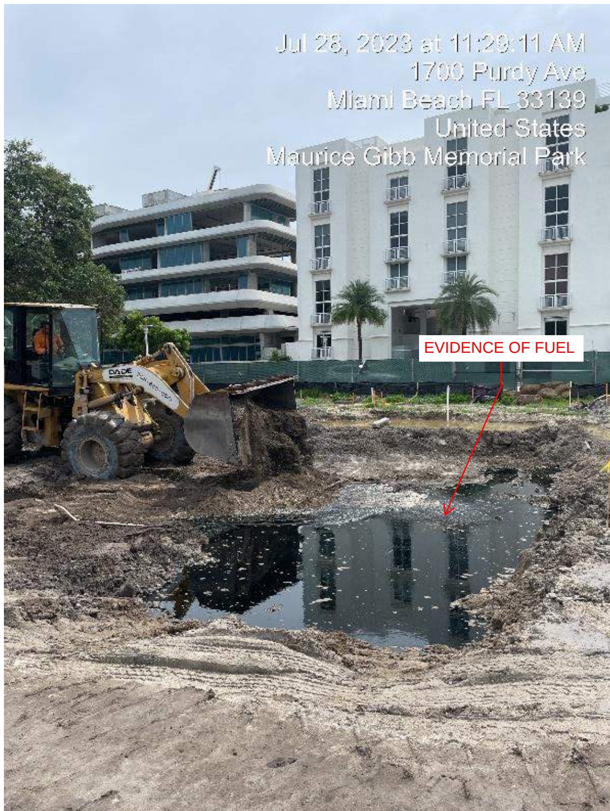
Area D: Fuel encountered signaled possibility of a underground fuel tank.
