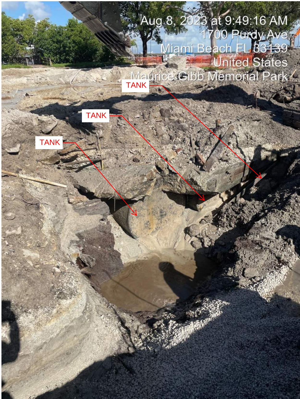
Area D: Underground fuel tank exposed.
