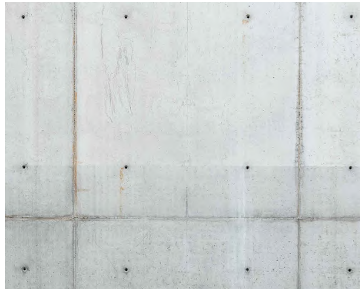
02 POOR CONCRETE FINISH
