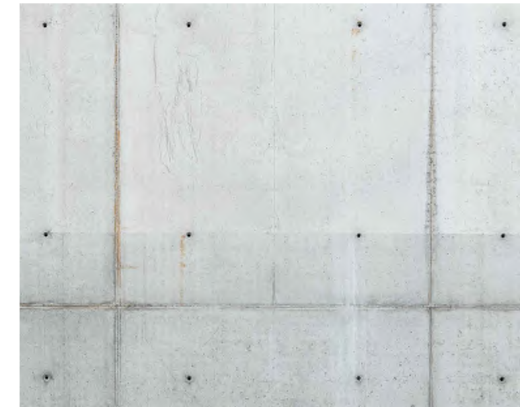
02 POOR CONCRETE FINISH
