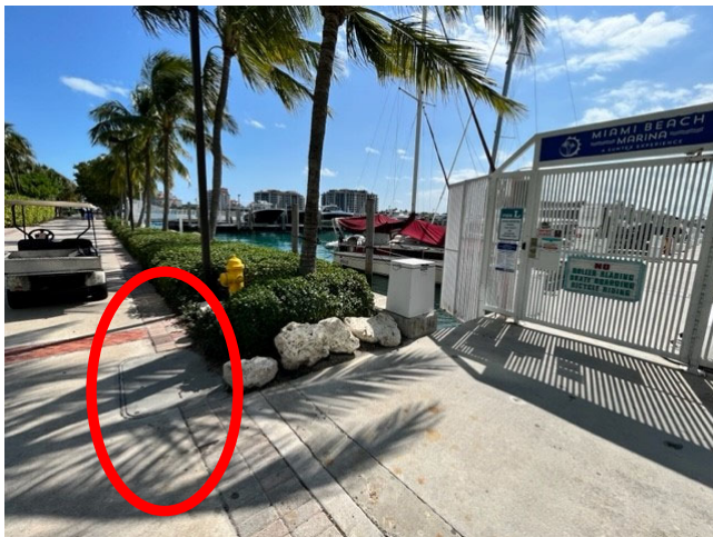
Junction Box at Head of Dock
