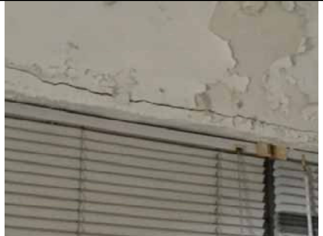
Apartment – cracking above window
