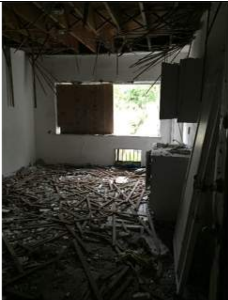
Apartment – exposed to elements
