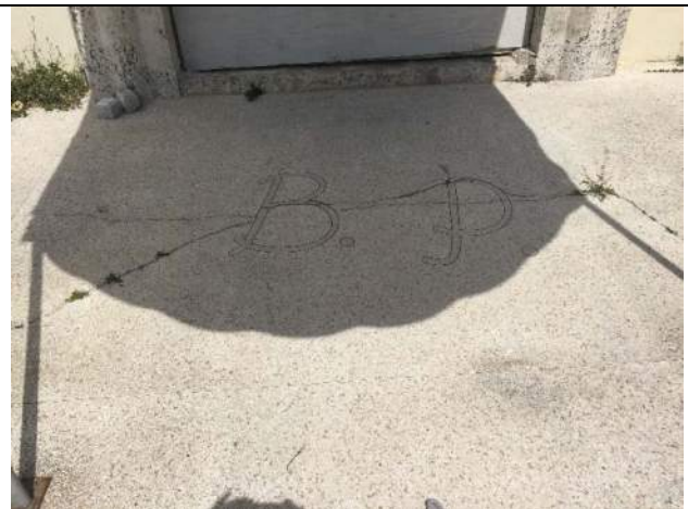
Main Entrance – Terrazzo cracked; logo “B.P.” Step up to lobby (ADA issue)
