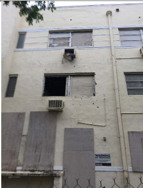
North Elevation Missing windows, water infiltration issue
