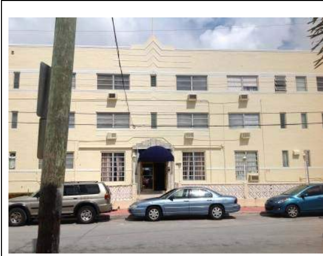
Park Avenue – Main Entrance. Small canopy. Long canopy connection still at wall
