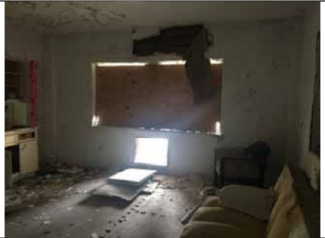
Apartment – exposed to elements
