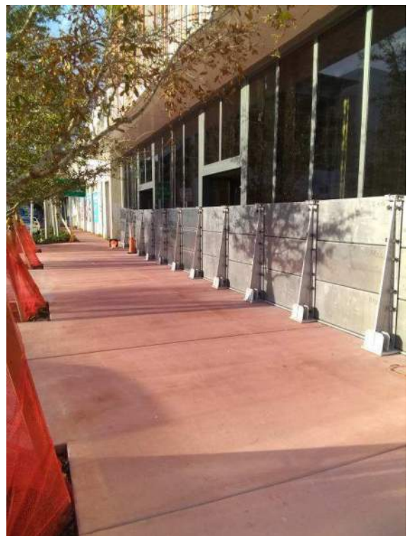
Window Wall – Perimeter Flood Protection Panels
