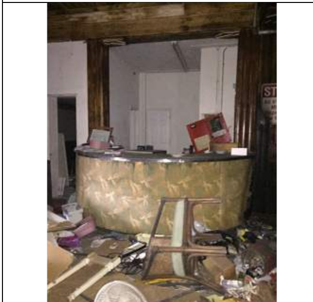
Lobby – desk, fire damage on right in image
