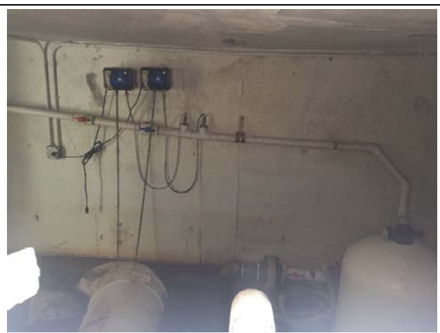
Pool Equipment Room - below pool deck
