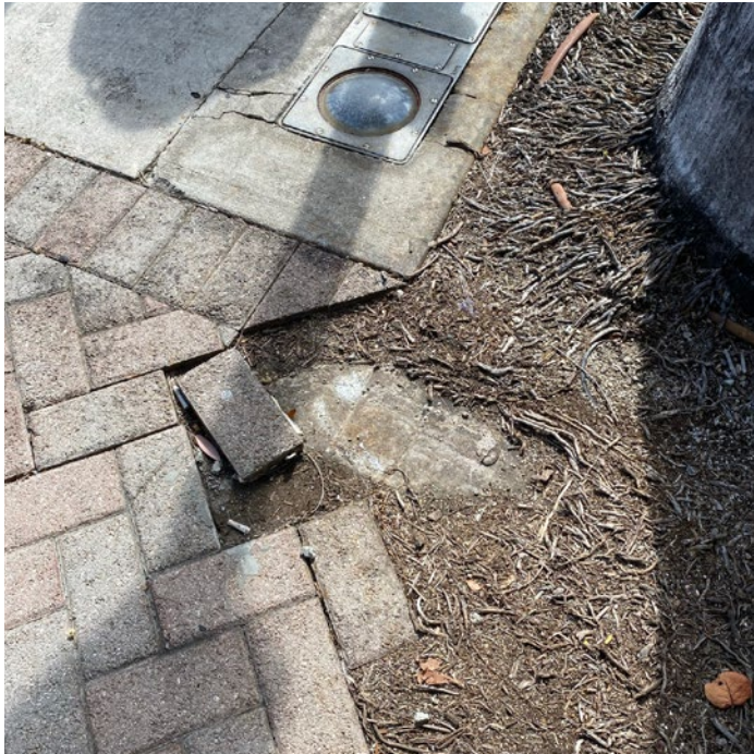
LOOSE CONCRETE PAVERS
