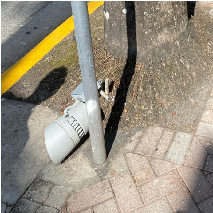
BROKEN LIGHT FIXTURES
