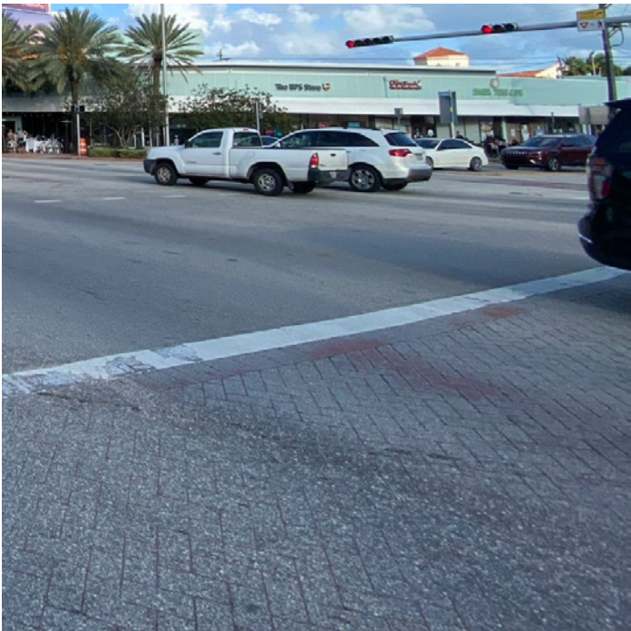
FADED CROSSWALK BRANDING
