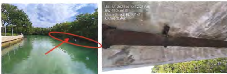
Figure A.2: Photo of canal where kayak launch is located and photo of pipe under bridge at 857 Michael Street.
