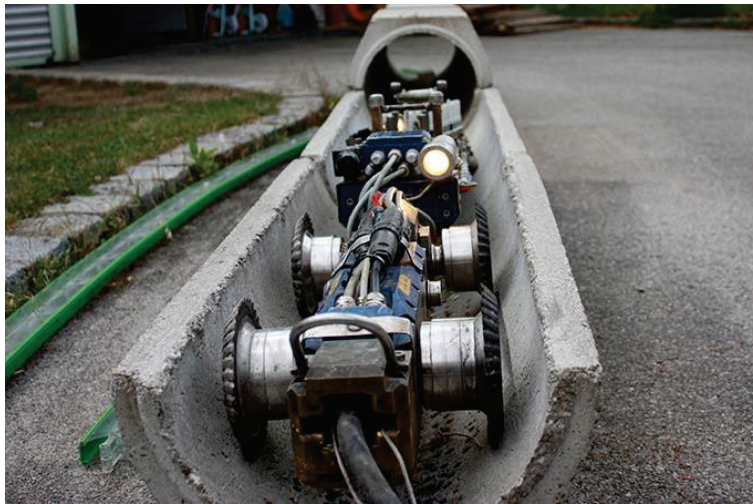
Figure 2-3: Current version of CableRunner robot used for installation of fiber optics in inaccessible sewers.
