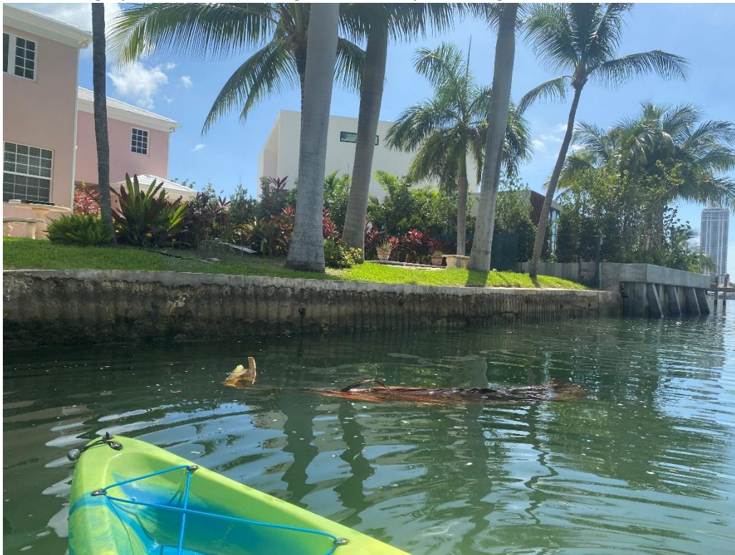
Photograph 4: View of existing seawall and structure and neighboring seawall from the canal facing northeast.
