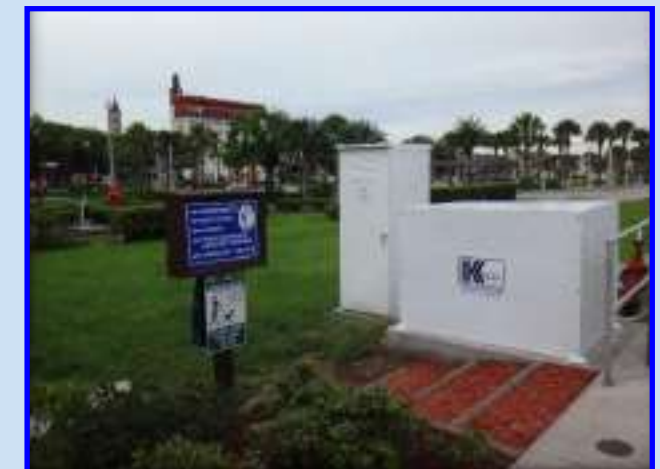
These photographs show examples of stationary sewage pump out facilities. These are located (from left to right) at City of Hallandale Beach, Mariner Cay in Martin County, Titusville and Saint Augustine.
