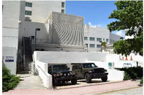
Fig. 126. View of areaway to lower level parking and stairs to mechanical area, July 2021.
