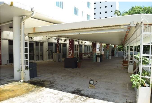
Fig. 138. Detail of area under canopy attached to east elevation of Cromwell, July 2021.
