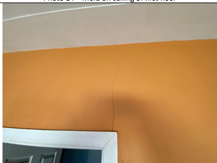
Photo 16 – Plaster cracking over door indicative of settlement
