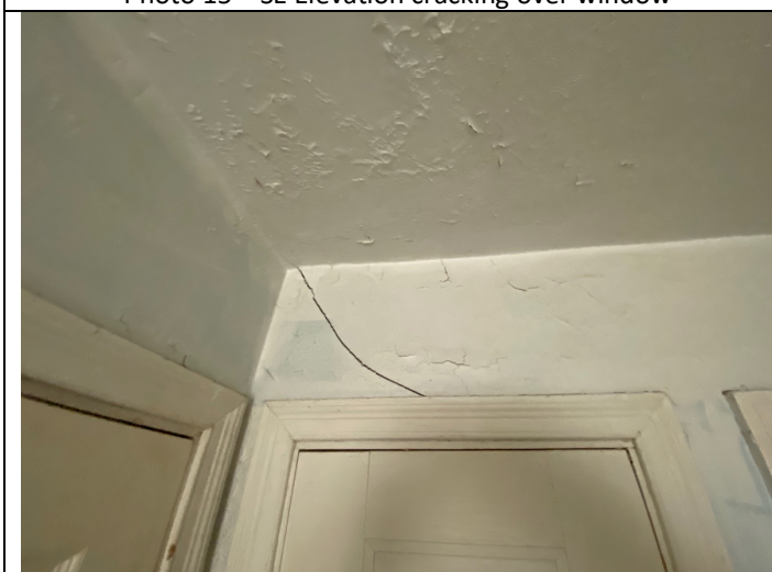
Photo 17 – Plaster cracking over door indicative of settlement
