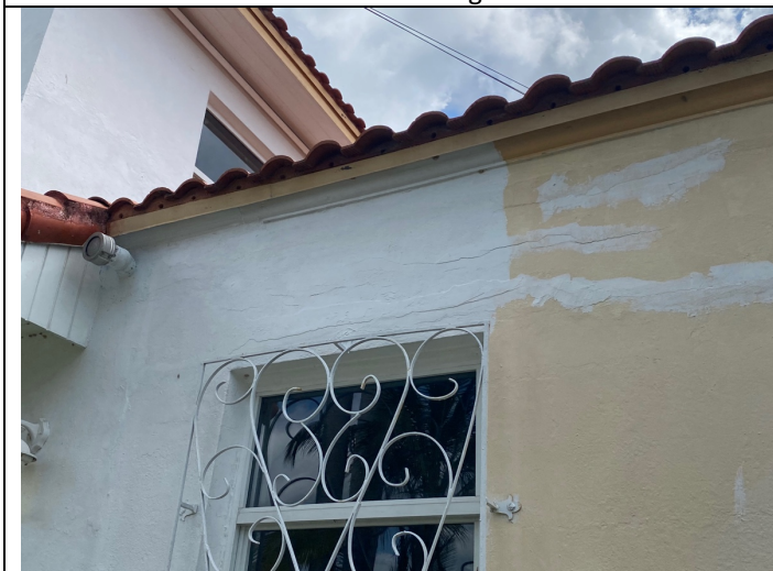
Photo 11 - West Elevation, concrete spalling
