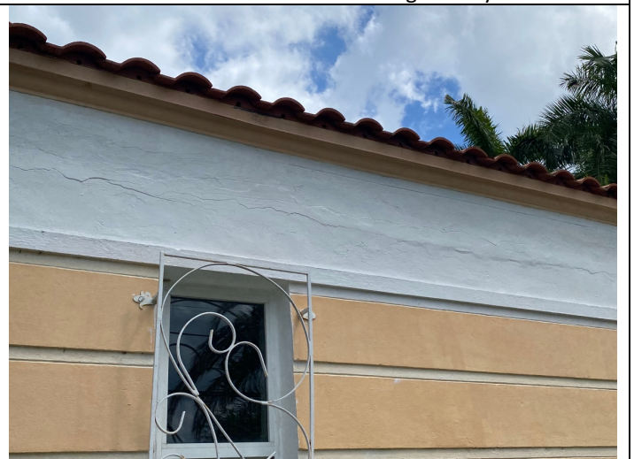
Photo 10 – Concrete spalling on SW elevation
