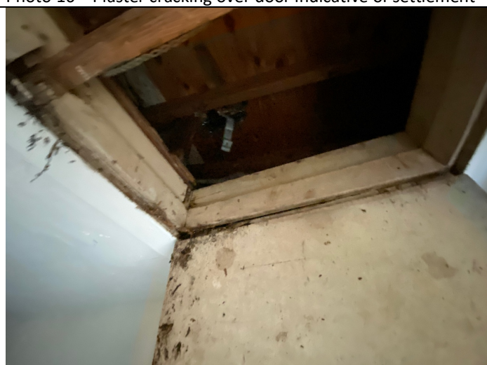
Photo 18 – Wood Damage of 2 nd floor
