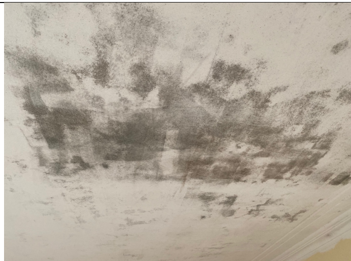
Photo 14 – Mold on ceiling of first floor
