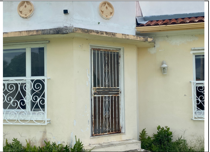
Photo 8 – NW corner beam cracking over eyebrow
