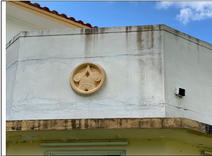
Photo 7 - North East Elevation wall and beam cracking
