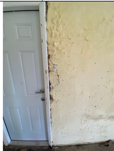
Photo 24 – Moisture damage on walls
