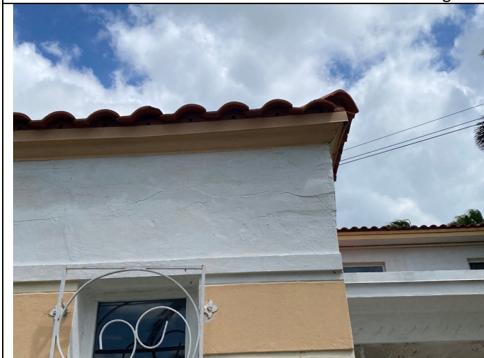
Photo 9 - Concrete Cracking SW elevation
