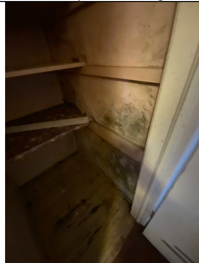
Photo 22 – mold presence in the second floor
