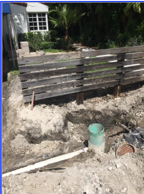
Figure 2. Photographs a whistleblower sent to DERM Sept. 20, 2018 that resulted in the discovery of more than 80 unpermitted drainpipe or stubs out in the right-of-way and the agency's enforcement action against the City
