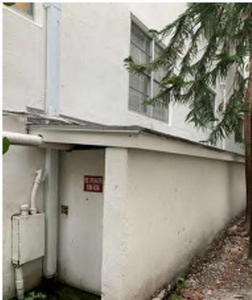
7 THE SOUTH SEAS - FIRE PUMP ROOM
