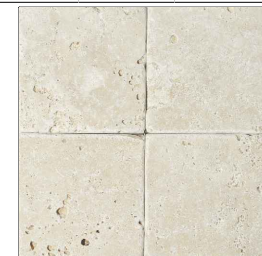
STONE CLADDING TO BE REPAIRED AND RESTORED
