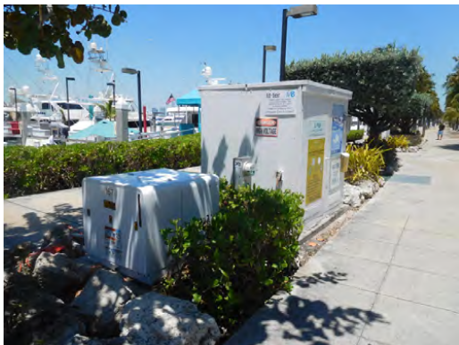
PHOTO #29 ELECTRICAL TRANSFORMER
