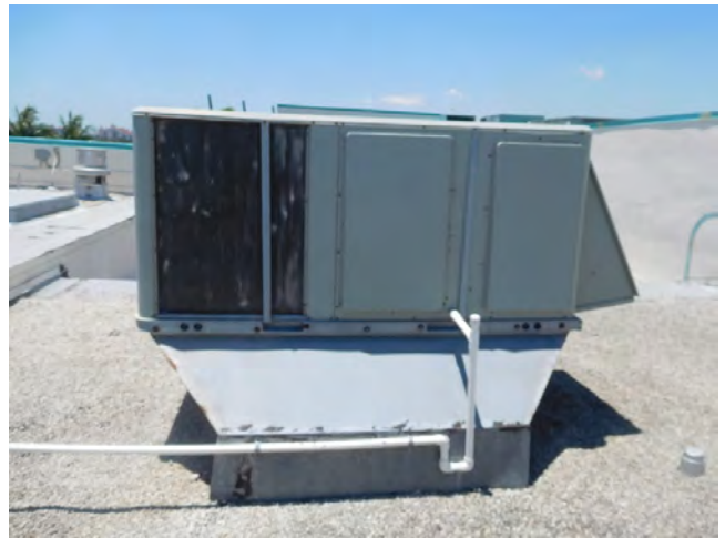
Rooftop packaged unit
