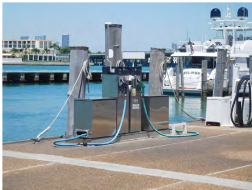
PHOTO #17 FUEL DISPENSERS
