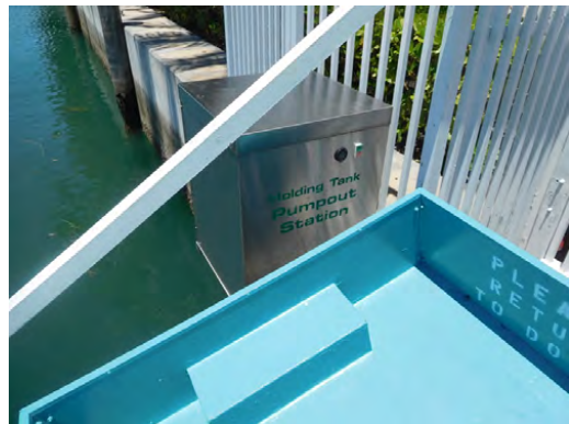
PHOTO #36 HOLDING TANK PUMPOUT STATION
