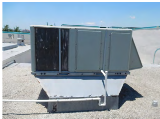
PHOTO #42 ROOFTOP PACKAGED UNIT
