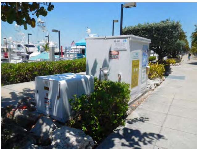
Electrical transformer (typical)
