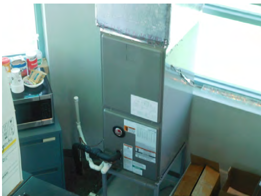
PHOTO #41 AIR HANDLING UNIT
