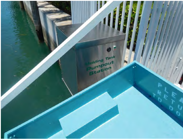
Holding Tank Pumpout Station
