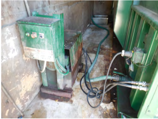
PHOTO #31 TRASH COMPACTOR HYDRAULIC EQUIPMENT
