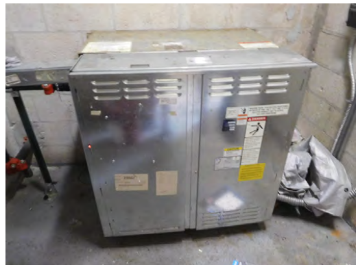
PHOTO #30 ELEVATOR EQUIPMENT
