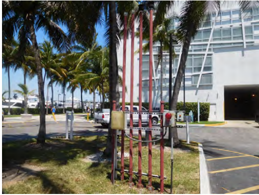
PHOTO #25 VENT PIPES
