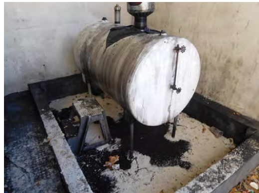
PHOTO #28 USED OIL AST
