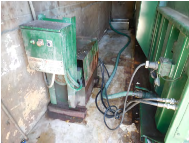
Trash compactor hydraulic equipment
