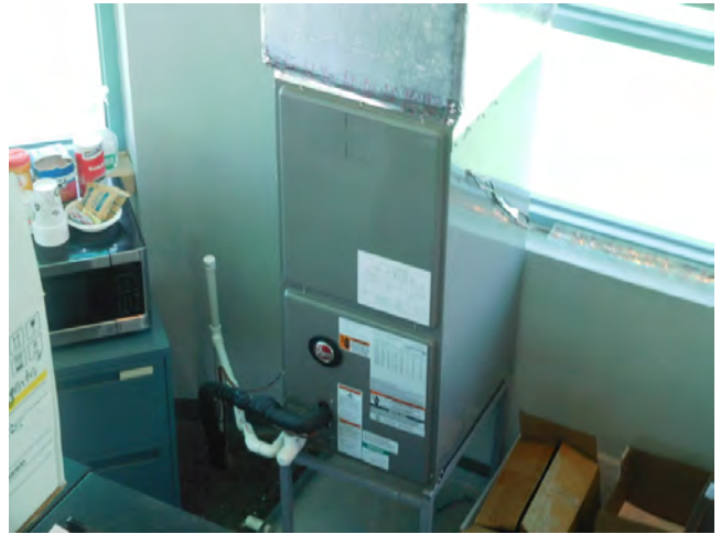
Air handling unit
