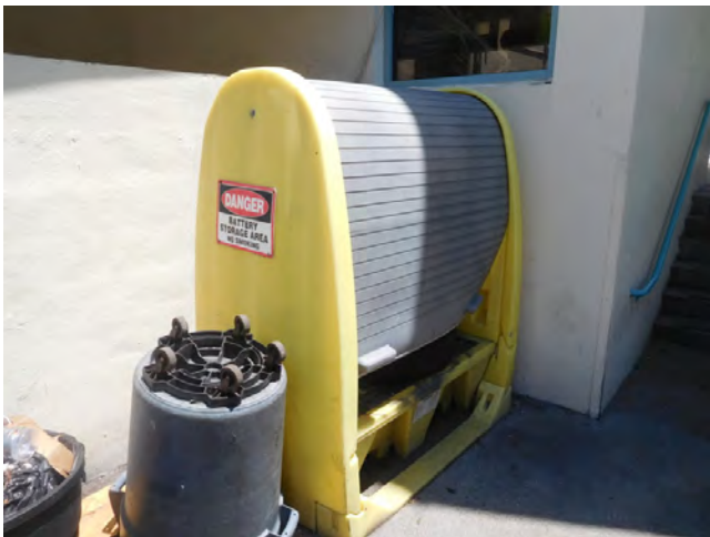
Used battery enclosure
