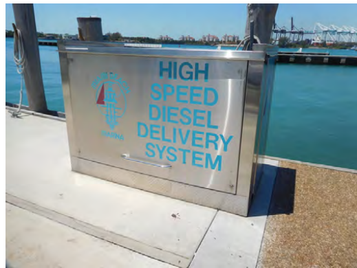
PHOTO #18 HIGH SPEED FUEL DISPENSER
