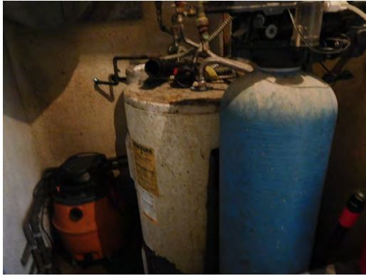
PHOTO #43 WATER HEATER
