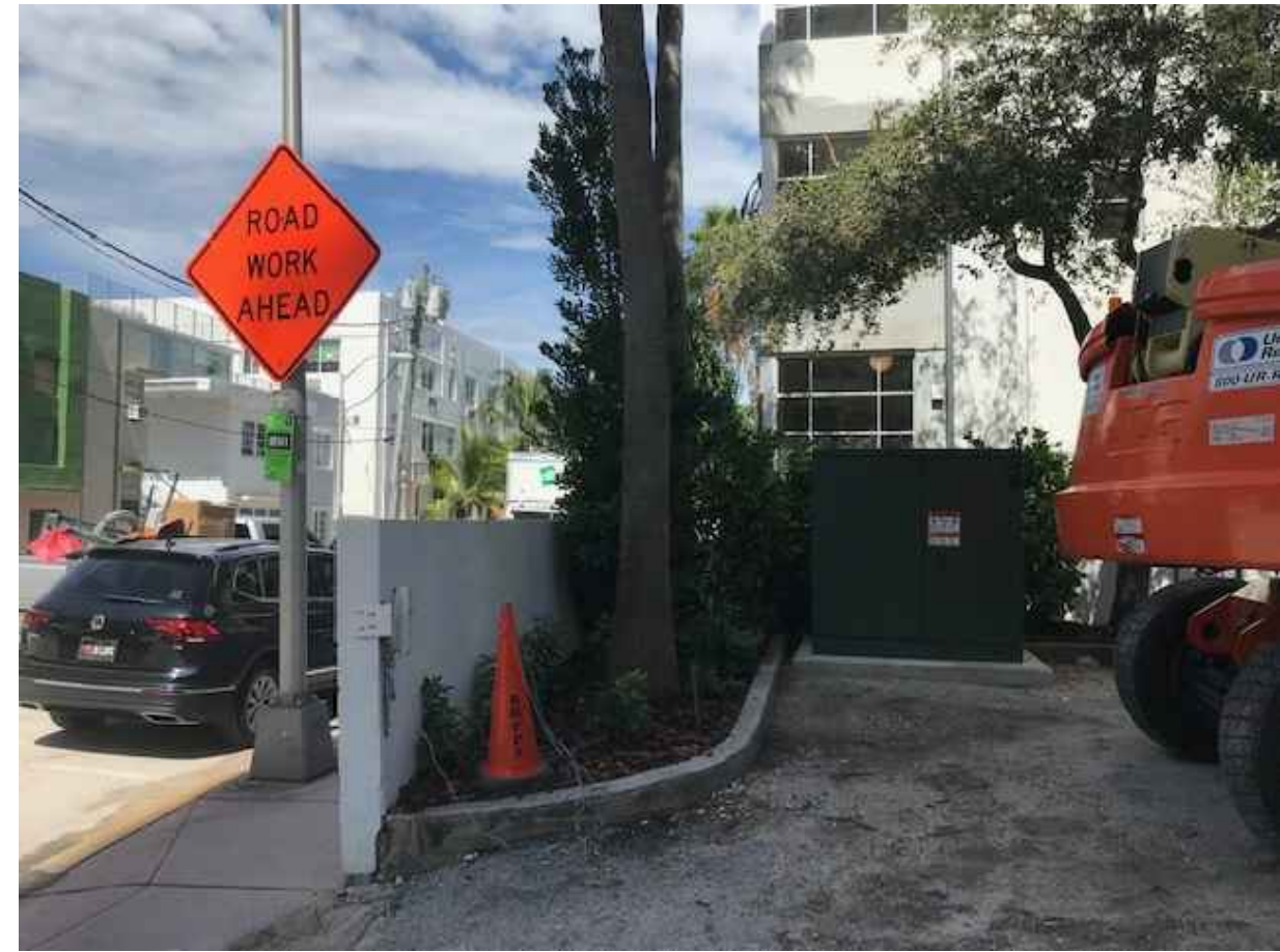
VIEW OF TRANSFORMER FACING WEST
