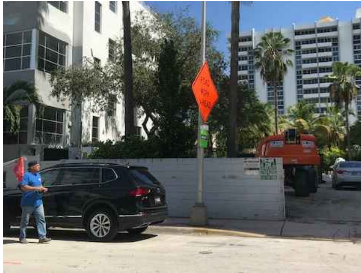
VIEW OF TRANSFORMER FACING NORTH
