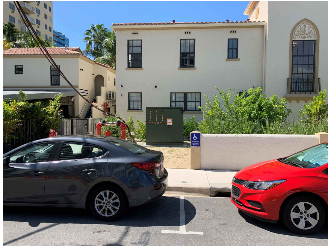
VIEW 1 OF ADJACENT GENERATOR HOTEL ELECTRICAL TRANSFORMER ALONG 31ST STREET
