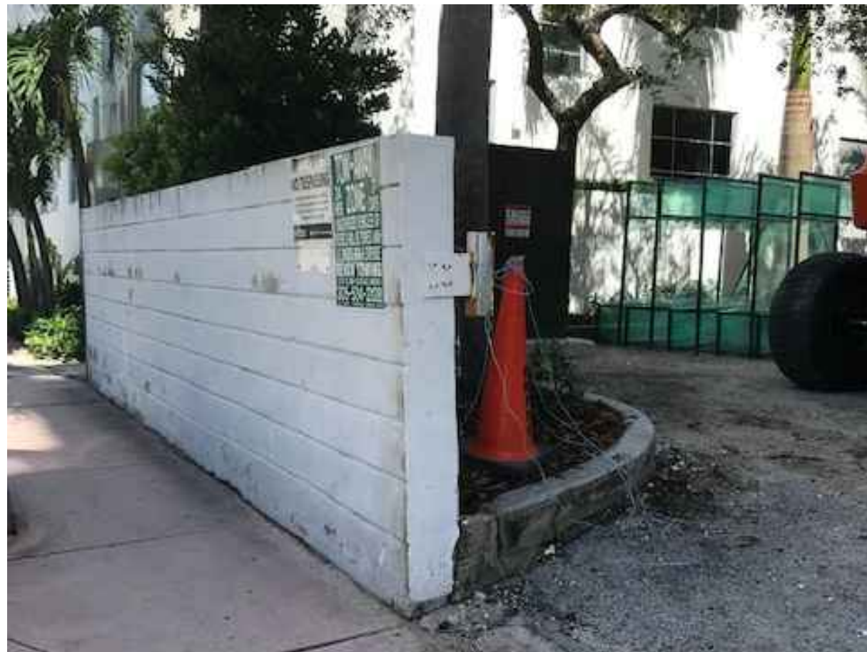
VIEW OF TRANSFORMER FACING NORTHWEST
