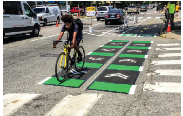
The two-way protected bike lane featured innovative conflict zone and intersection markings, to ensure that motorists knew to look for bike traffic before turning onto or from Broad St.
