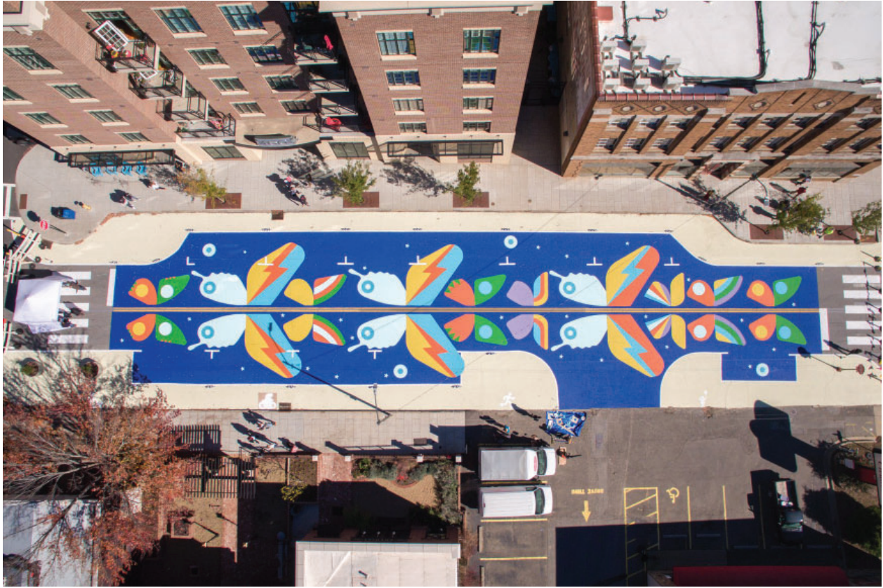
Using large-format stencils (over 20 separate pieces), Street Plans and volunteers laid out the design created by local artist Jenny Fares. The 6,000 square foot mural took 1.5 days to lay out and paint.
