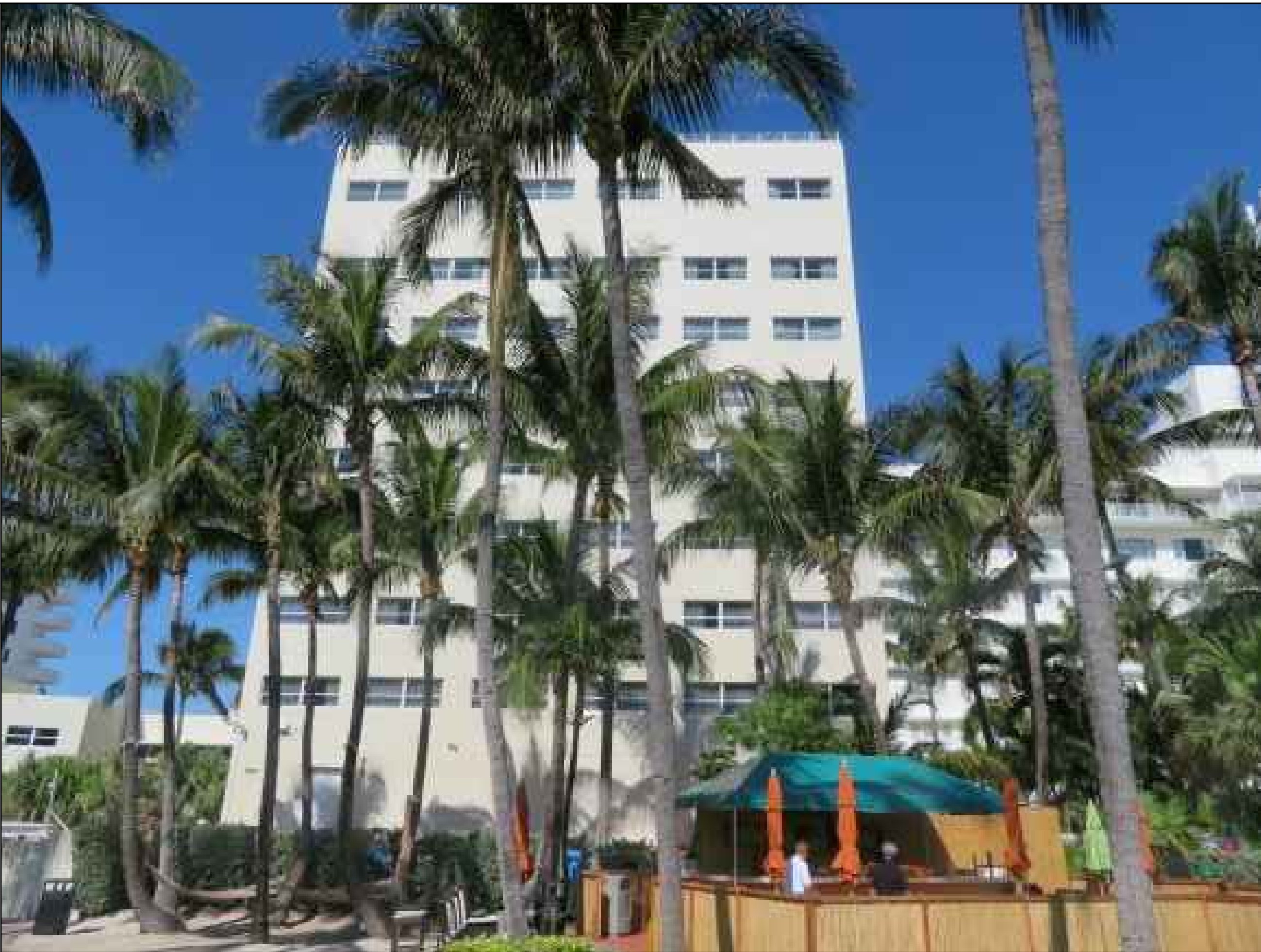
4 EAST ELEVATION, VIEW FROM THE BOARDWALK NOT IN SCOPE OF WORK SEE ARCHITECTURAL ELEVATION, SHEET A-4.3 PHOTO, DATED 4.3.2019
